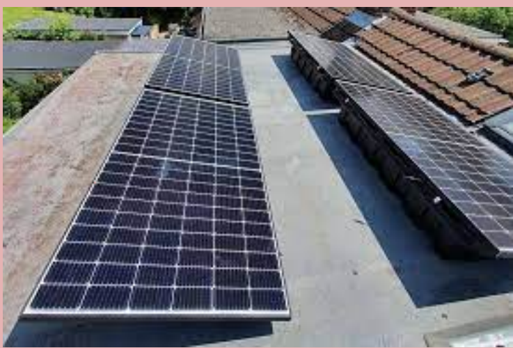
Photovoltaic Panels on Single Ply membrane
