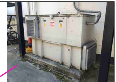
Telecomms. Backup generator and tank
