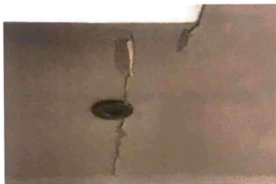
Crack to ceiling in kitchen / living area.
