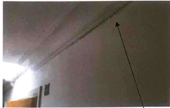
Coving separation in hallway.
