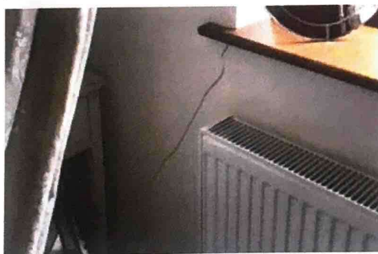
Crack to left of radiator to front bedroom window.
