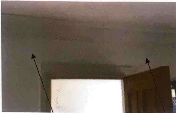
Cracks to plastered wall entrance to kitchen living room.
