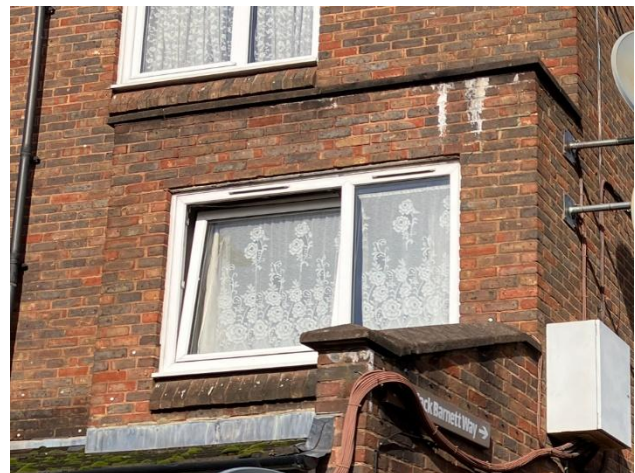
Photo 18. Efflorescence staining beneath coping stones.
