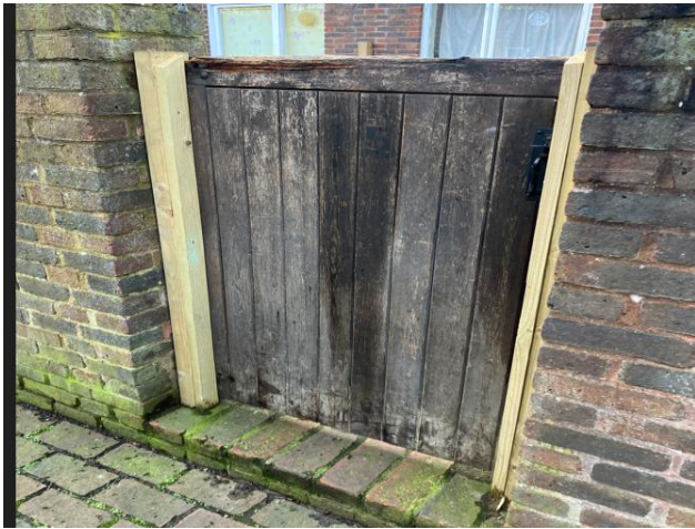
Photo 15. Localised rot to timber gates.
