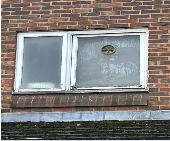
Photo 7. Deteriorating timber windows.
