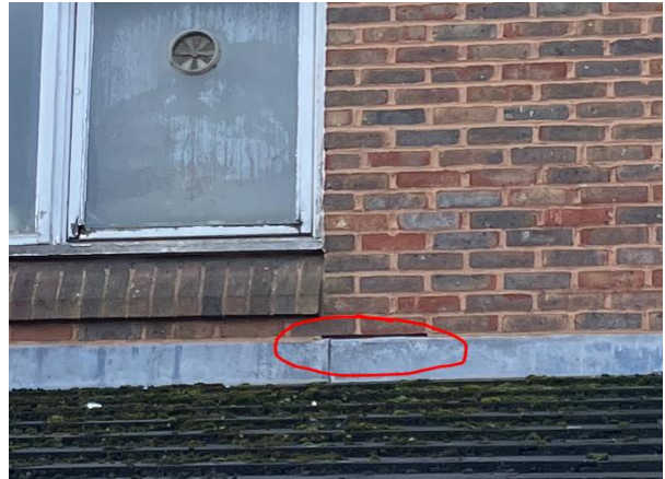
Photo 14. Receded mortar joints to the front elevation.
