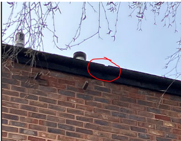
Photo 11. Cracks to the guttering (front elevation)
