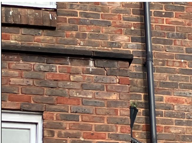
Photo 17. Cracking to rear bay projection.
