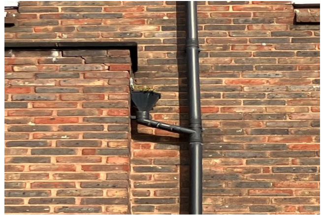
Photo 10. Blocked hopper to the rear elevation.
