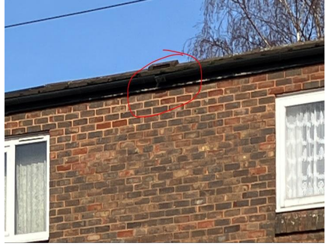
Photo 8. Undulated and loose guttering.
