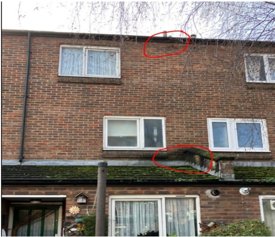
Photo 9. Ongoing leak to front elevation.
