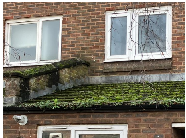
Photo 6. Moss build up and staining to coping stones.
