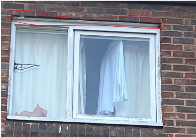
Photo 13. Surface rust to metal lintels.
