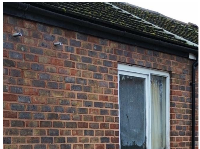
Photo 12. Undulated guttering to the front elevation.
