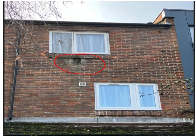
Photo 4. Staining to brickwork (nr.20)
