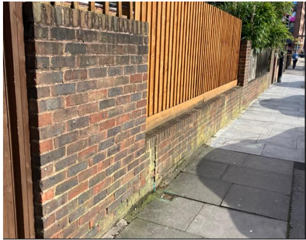
Photo 16. Expansion cracking to boundary wall.
