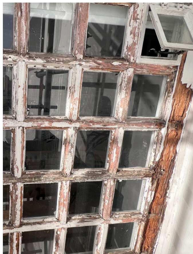
Loggia window - timber frame in state of serious disrepair. Note steel-framed opening lights in top corners (to be retained and reinstalled in replacement window).
