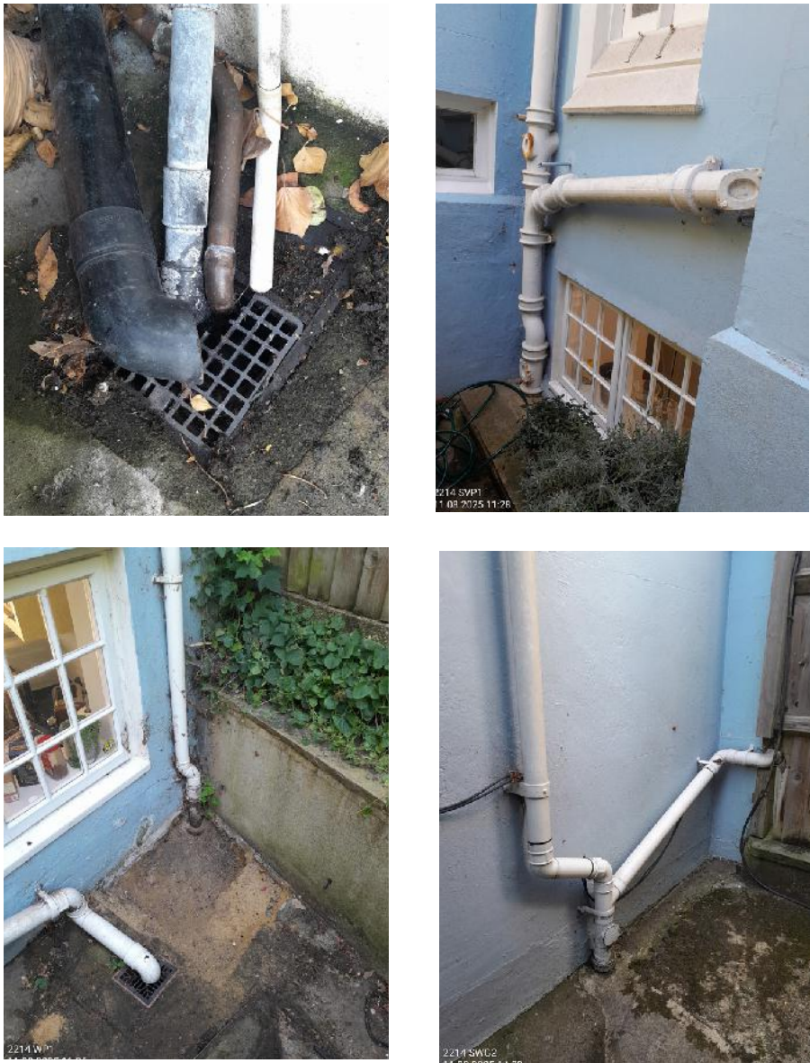
Site images showing unsightly pipes on the rear elevation
