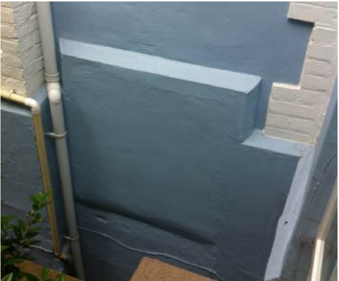
Eastern lightwell - change of surface texture at missing window
