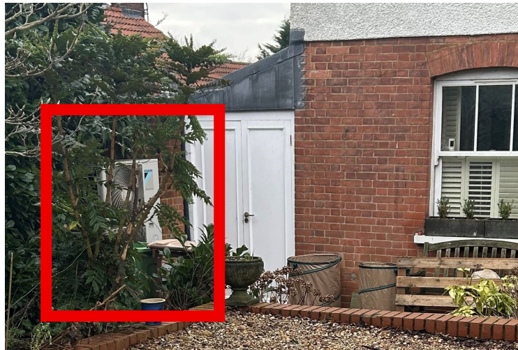
Image 2: External unit on No.9 Southern Road
