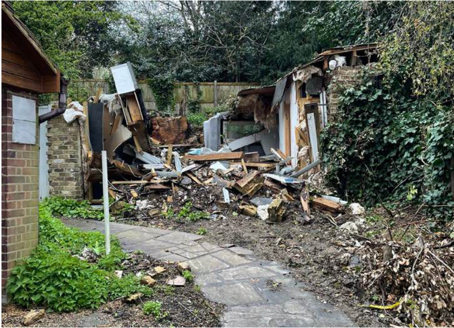
Studio Annexe after damage from fallen tree
