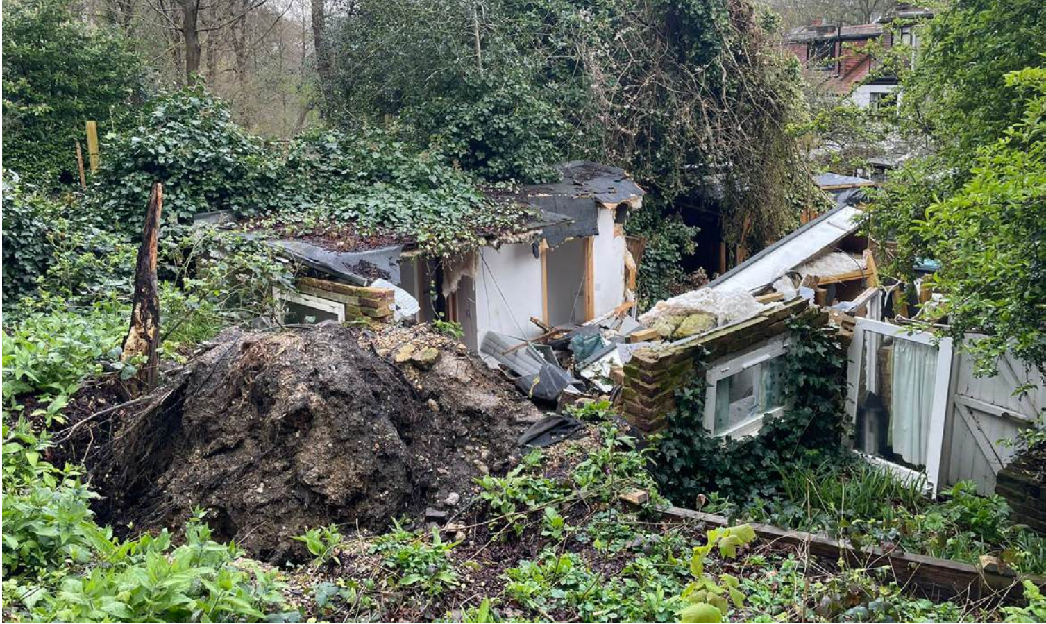
Studio Annexe after damage from fallen tree
