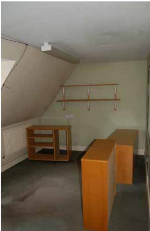
Extremely restricted headroom at first floor
