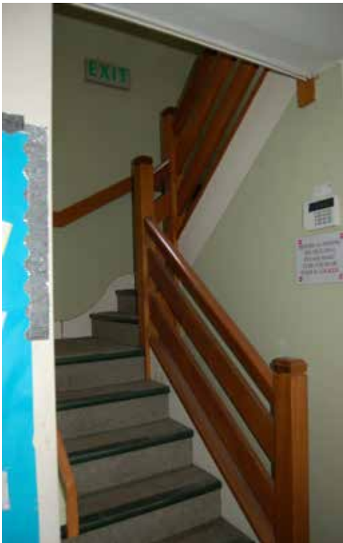
Restricted stair access
