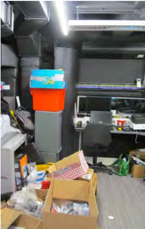
Inappropriate support facilities
