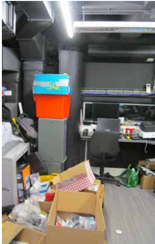
Inappropriate support facilities
