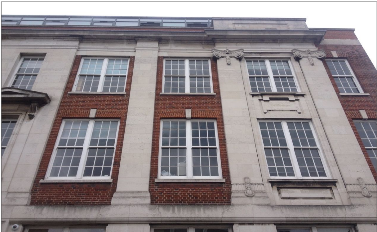
Existing stonework and brickwork requiring renovation
