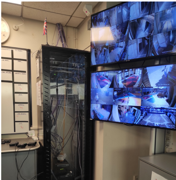
Figure 3: Equipment in Control Room
