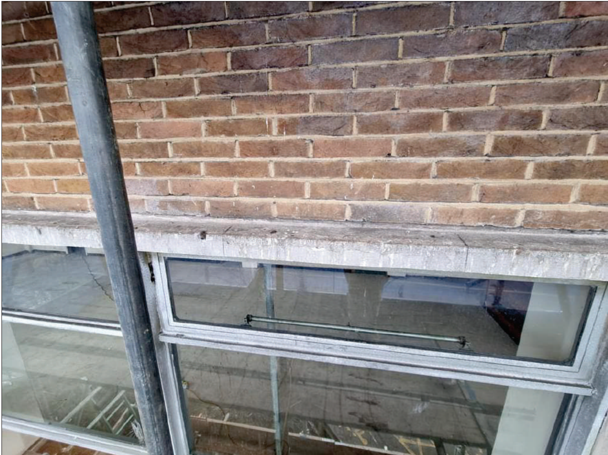
Pre-cast window head repair - before
