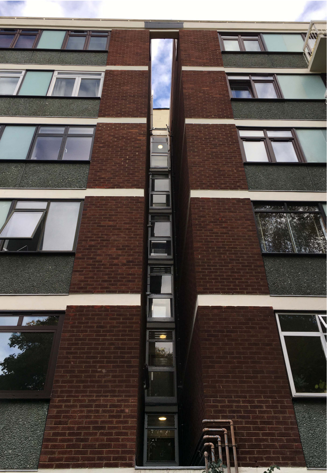
Side elevation showing inconsistency in the window frames within the same building
