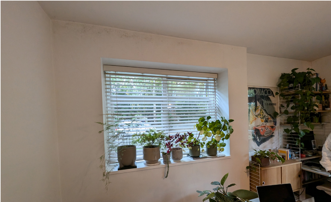
Photo of the existing window and balcony door showing poor condition of the frames and mould
