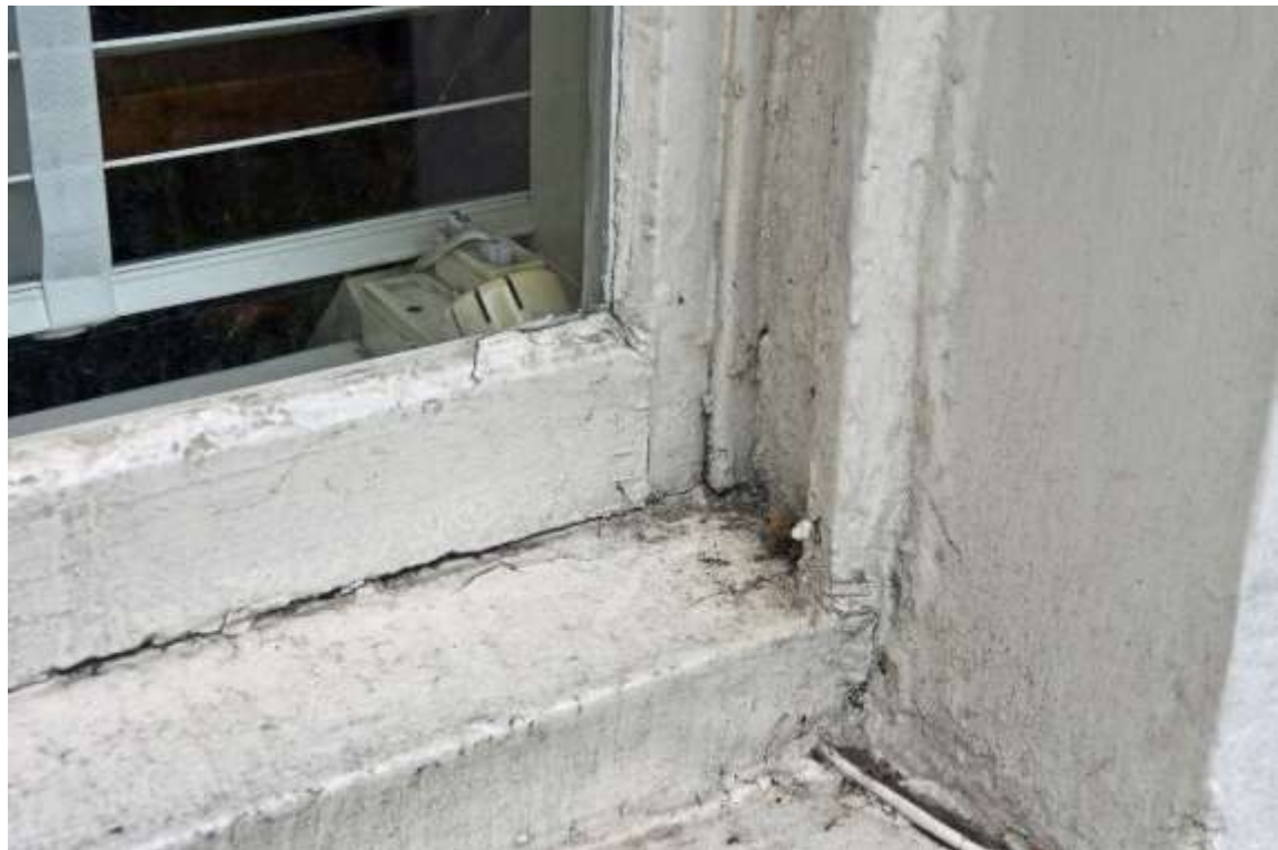
Figure 19: Detail of lower left window, areas of repainted and cracking paint visible.
