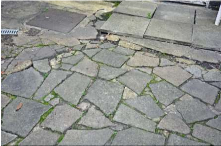
Figure 107: Current condition of rear garden patio paving by the garden access door. Taken 01.11.24.
