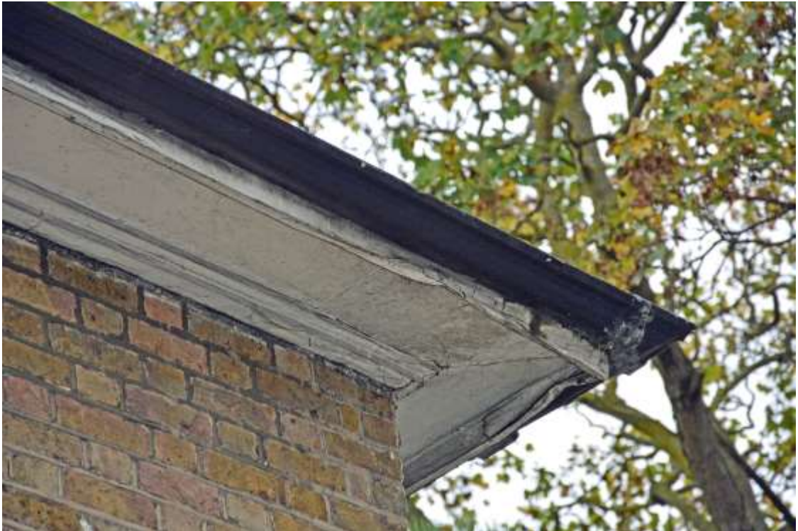
Figure 39: Existing condition of the soffits and fascia, right corner of the front façade.
