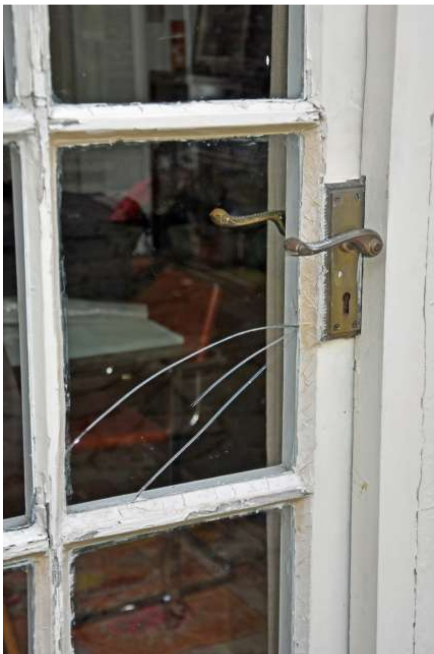
Figure 68: Detail photograph of cracked pane within the garden door on the rear elevation. Taken 22.10.24.
