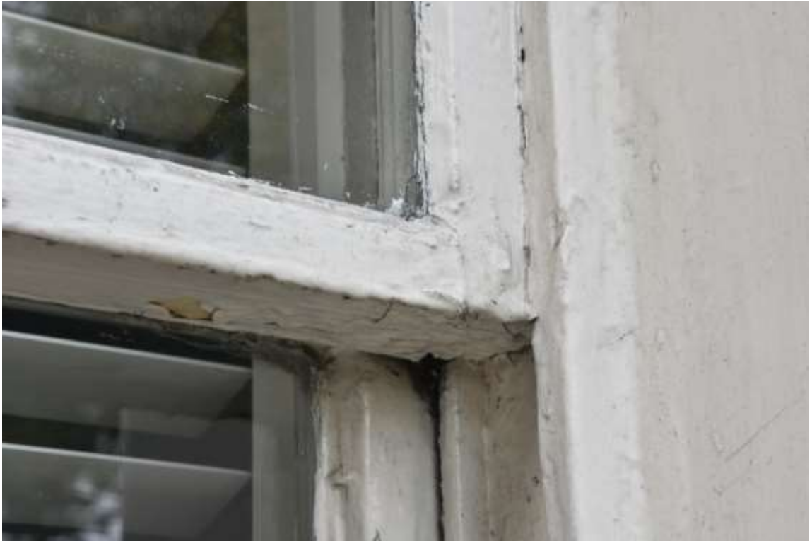
Figure 18: Detail of lower left window, thickened areas of repainted window visible.
