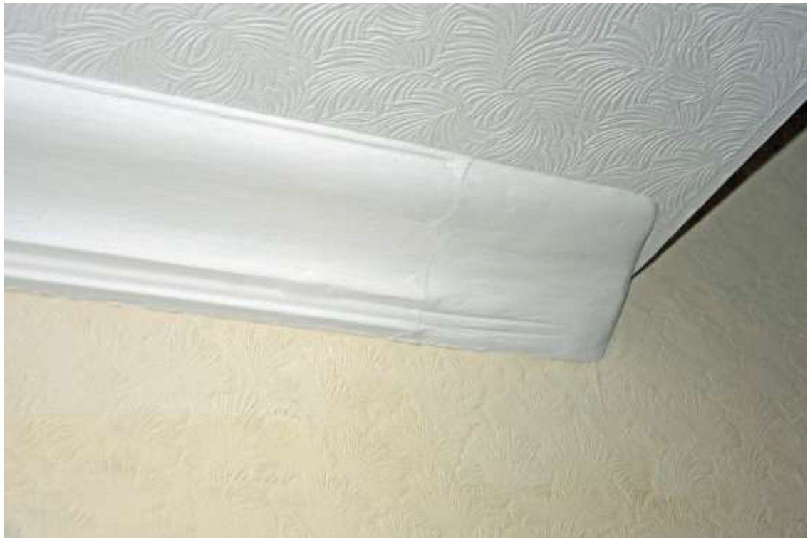
Figure 121: Detail Photograph of hallway coving, north wall. The original section to the left, with a smaller area of remoulding to the right adjacent to the double-height space. Taken 22.10.24.
