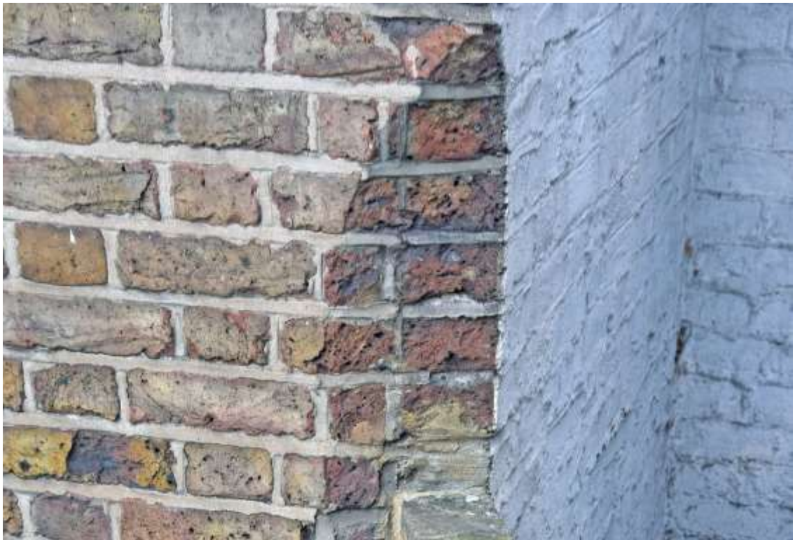
Figure 47: Detail of cut feature to the brickwork between the front façade and northern side elevation.
