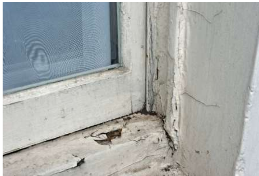
Figure 33: Detail of lower right window; areas of thickened/flaking paint visible.
