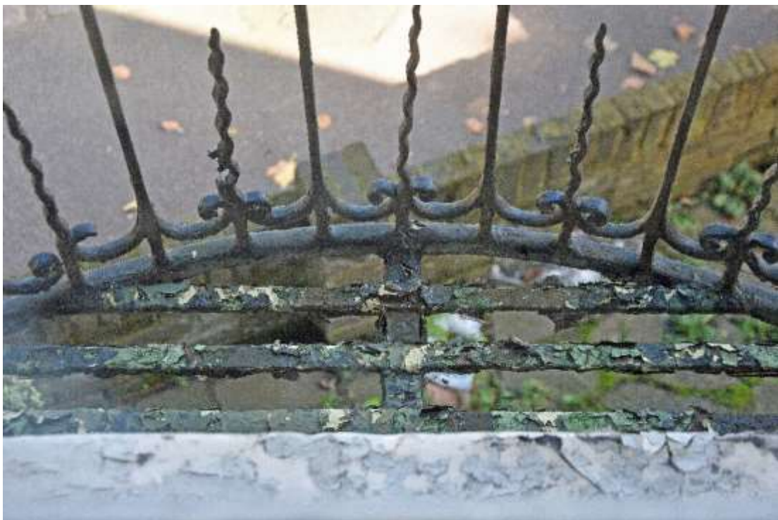
Figure 28: Detail of Upper Right window balconette, flaking paint visible. Damaged paint on the window frame visible in the foreground.
