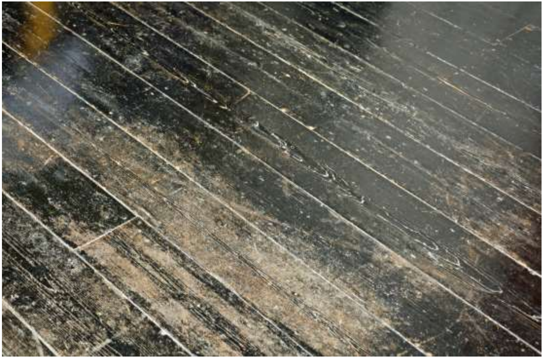
Figure 186: Photograph detailing the condition of the flooring in Area Q. Taken 01.11.24.
