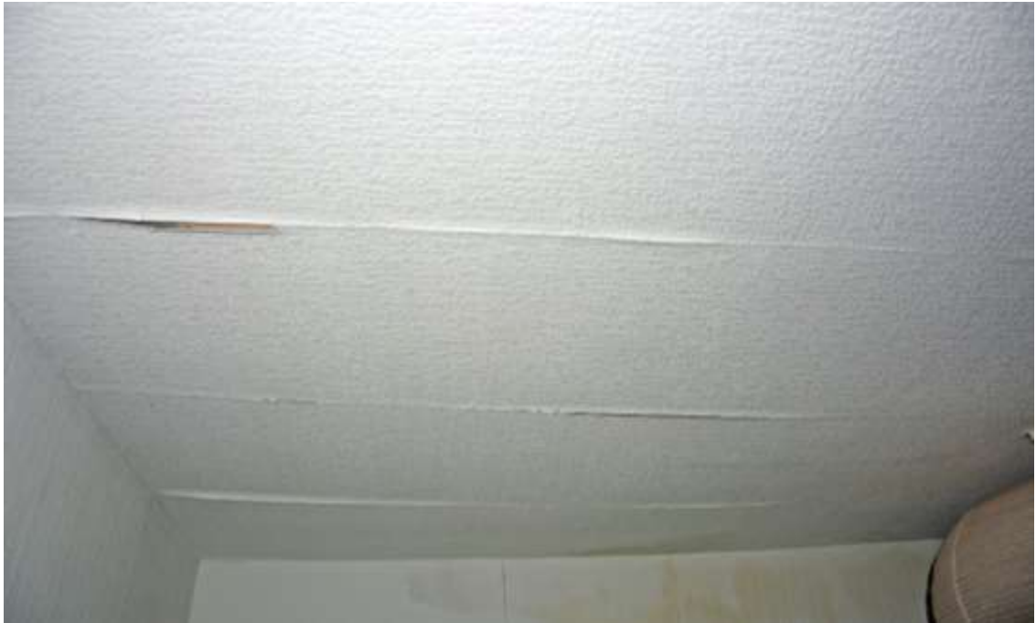
Figure 181: Detail Photograph of condition of ceiling wallpaper in Area P. Taken 01.11.24.
