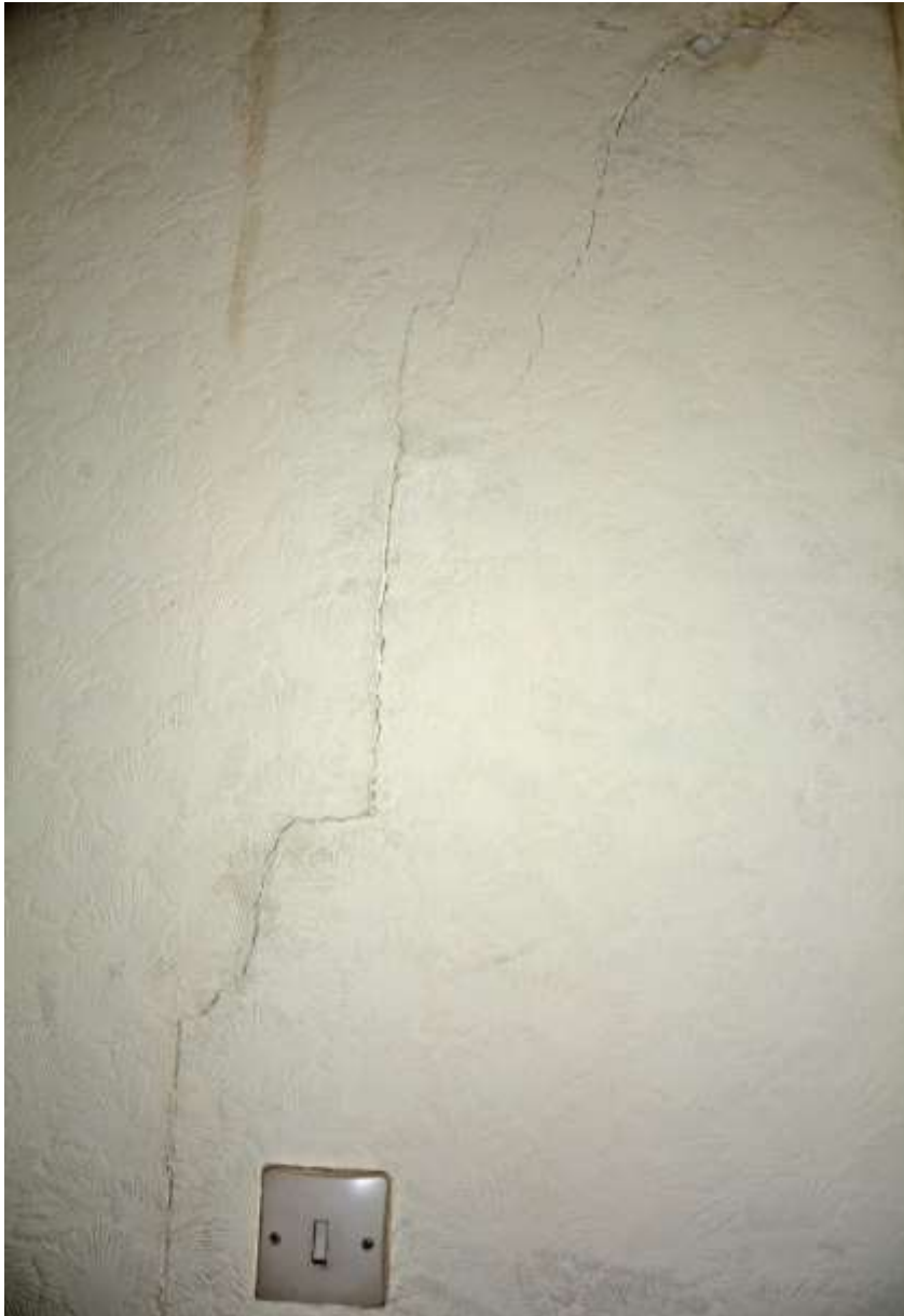
Figure 126: Detail Photograph of the existing wall directly to the right of the front door. Cracks visible in the wall and wallpaper. Taken 01.11.24.
