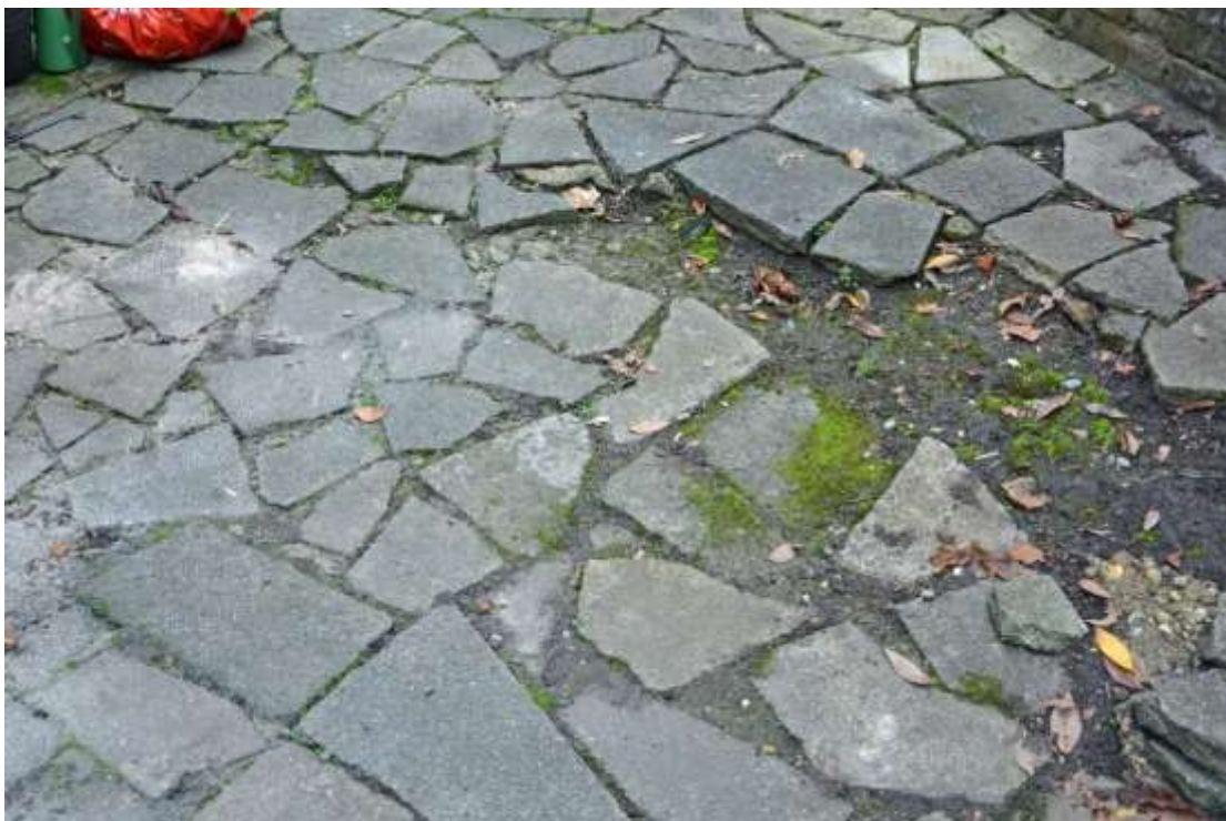
Figure 106: Current condition of rear garden patio paving. Taken 01.11.24.
