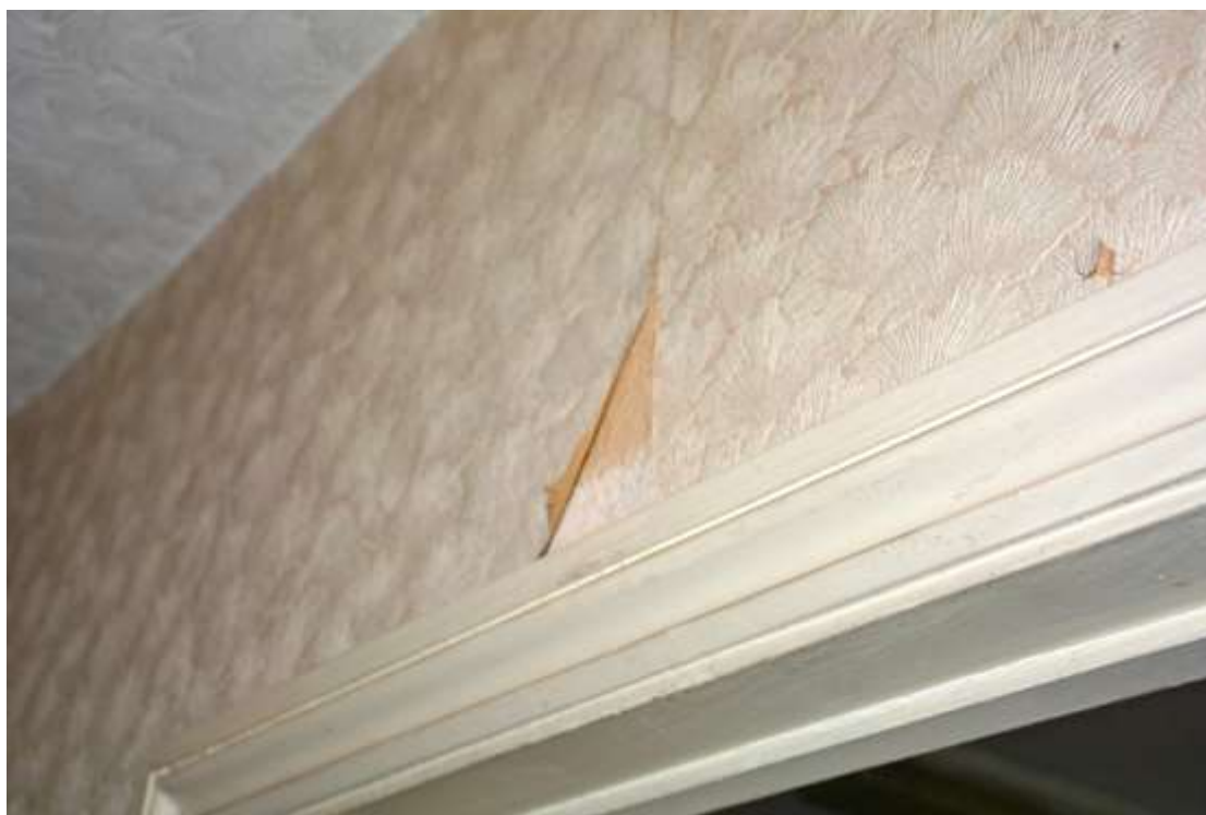
Figure 138: Detail Photograph of door frame and wallpaper condition in Area D. Taken 01.11.24.
