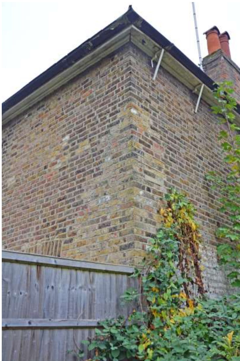
Figure 85: Photograph of the corner between the rear (west) and side (south) elevations with clear evidence of rebuilding. Taken 01.11.24.
