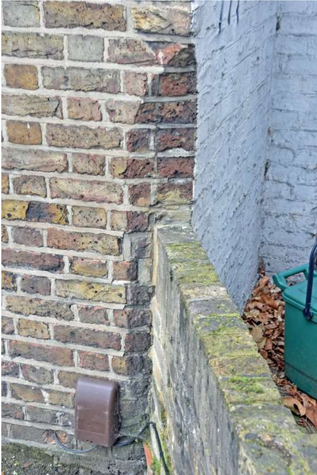
Figure 48: Overview of cut feature to the brickwork between the front façade and northern side elevation.
