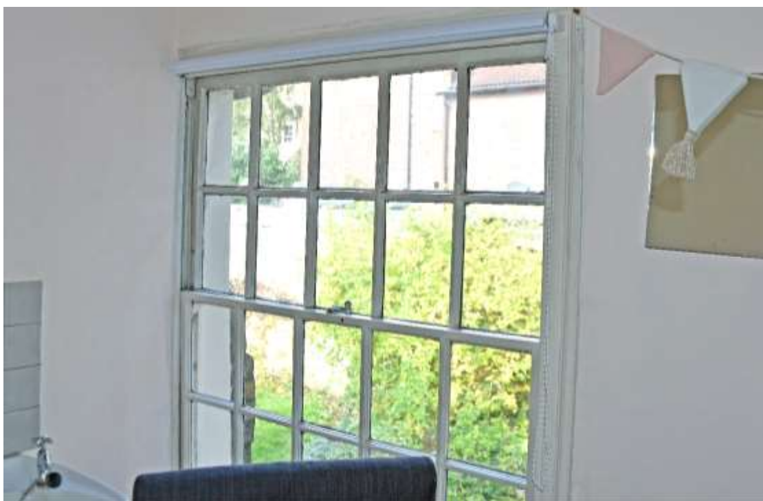
Figure 176: Photograph of window in Area O. Taken 22.10.24.
