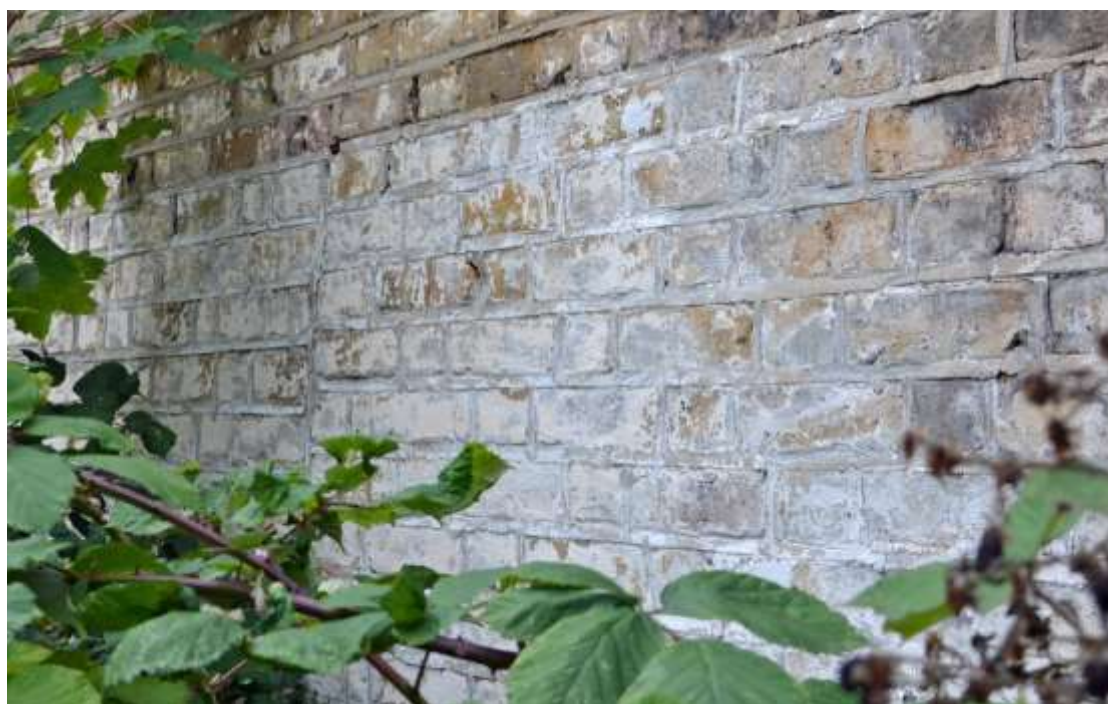
Figure 87: Detail Photograph of painted area within southern side elevation. Possible blocked opening visible to the right of the image. Taken 01.11.24.
