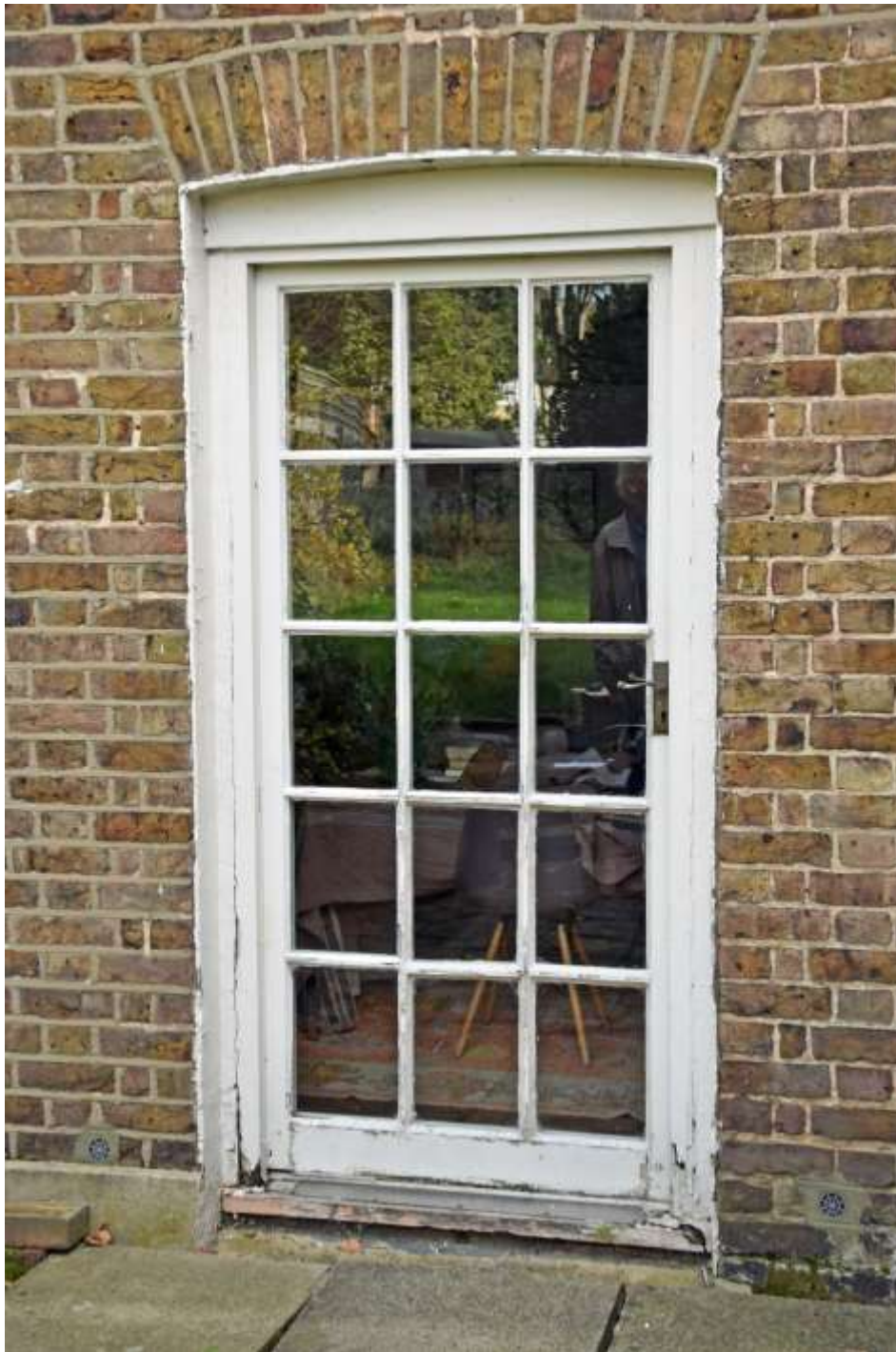
Figure 67: Overview Photograph of Garden Access door on rear elevation. Taken 22.10.24.
