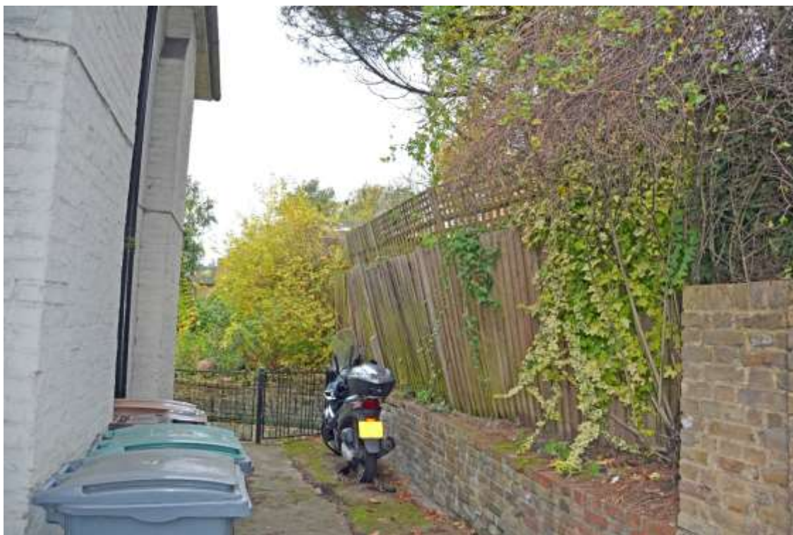
Figure 103: Overview of side access area and damaged fence. Taken 01.11.24.
