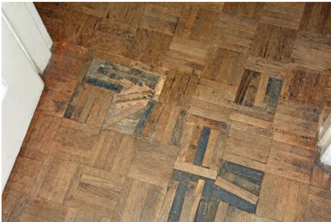
Figure 123: Floor condition within the hallway (Area B). Entrance to Area C. Taken 01.11.24.
