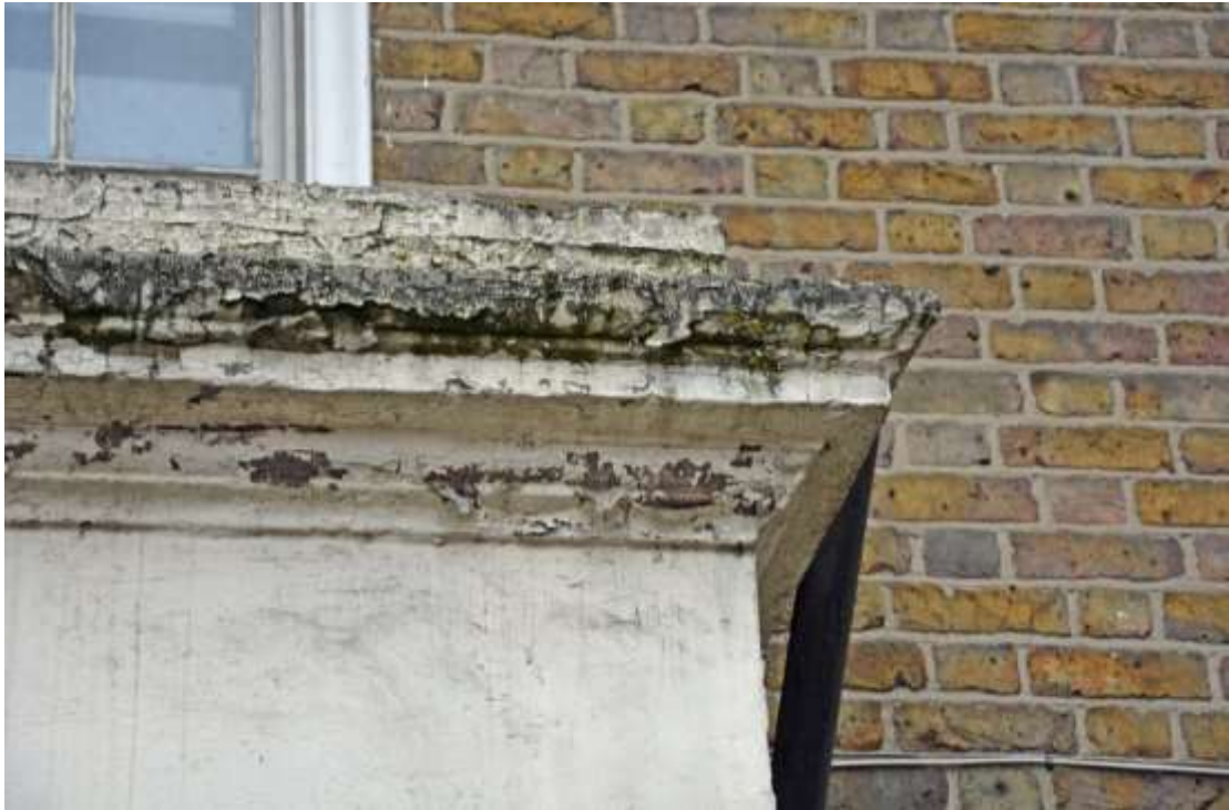
Figure 35: Detail of upper right corner of front porch, heavily damaged external rendering.
