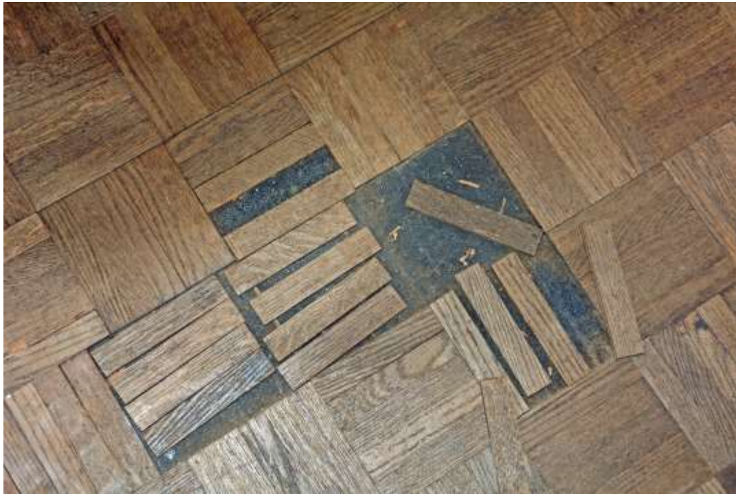
Figure 122: Floor condition within the hallway (Area B). Taken 01.11.24.
