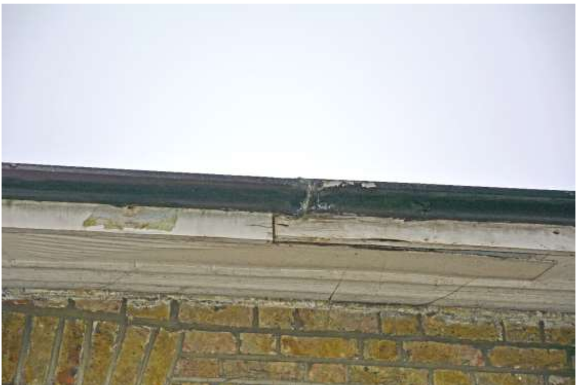
Figure 40: Existing condition of the soffits and fascia, to the rear of the property.
