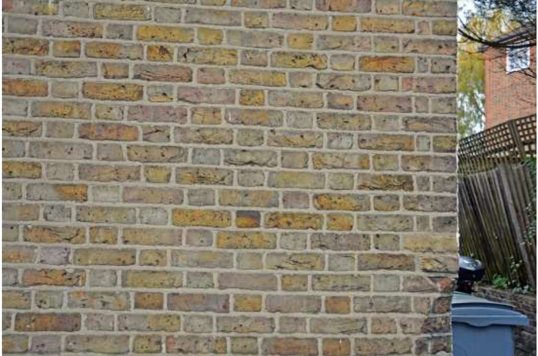
Figure 37: Condition of brickwork on the front façade of 9 Muswell Hill, right corner of the residence.
