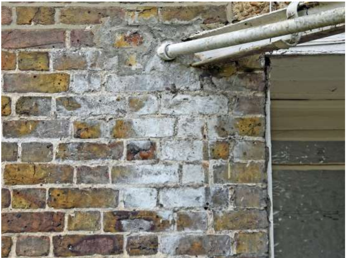
Figure 74: Detail Photograph of damaged brickwork due to the installation of the steel beams for the external stair case – rear elevation. Taken 22.10.24.
