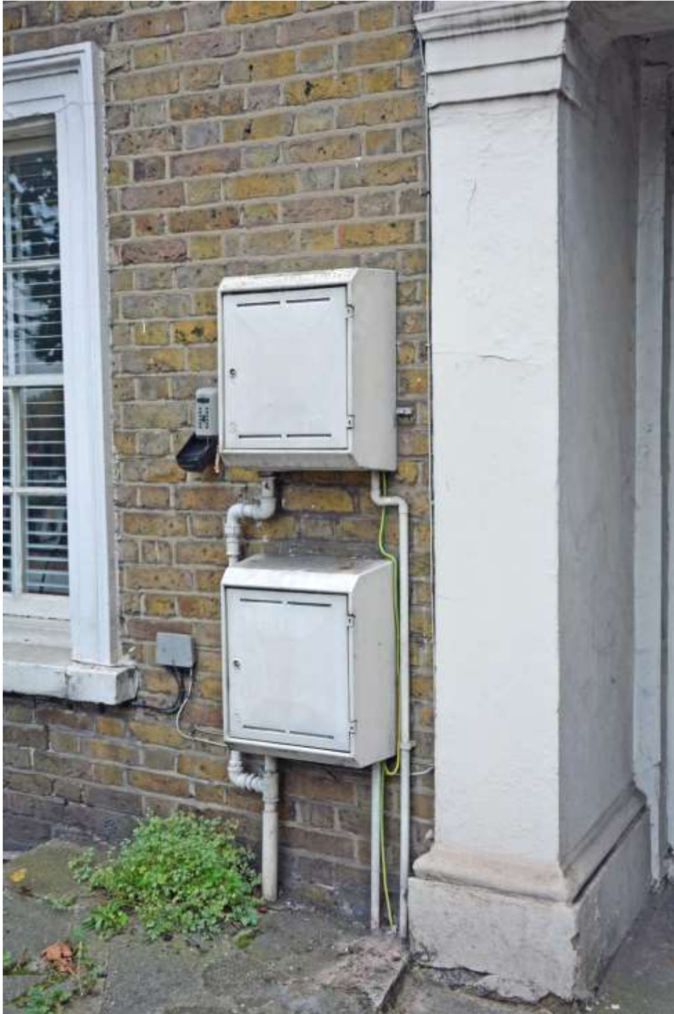
Figure 41: Utilities installed on the front face of 9 Muswell Hill.
