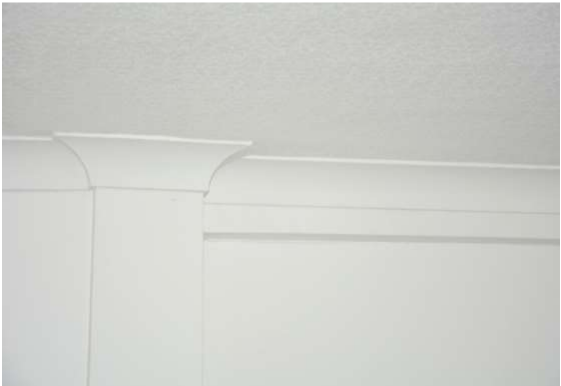
Figure 142: Detail Photograph of coving within Area E – southern wall. Taken 01.11.24.
