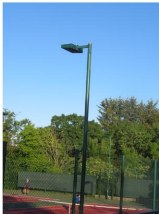
Existing columns and box luminaires with horizontal cut off (court 4)
