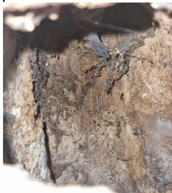
Plate 17: Large and extensive cavity of T2. PRF-M bat roost potential.
