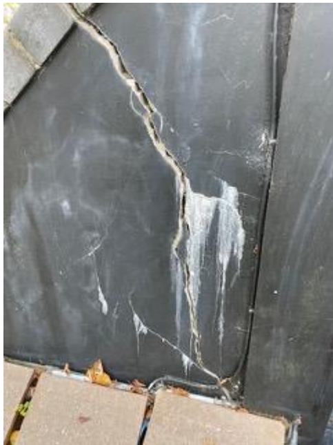
Image of front staircase cracking.
