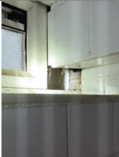
Photo 7 (24/04/2025): Building 1: Missing tiles leading to internal cavities in the bathroom.
