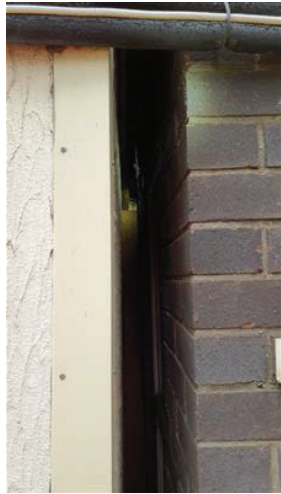
Photo 5 (24/04/2025): Building 1: 20 cm gap between extension and original building.
