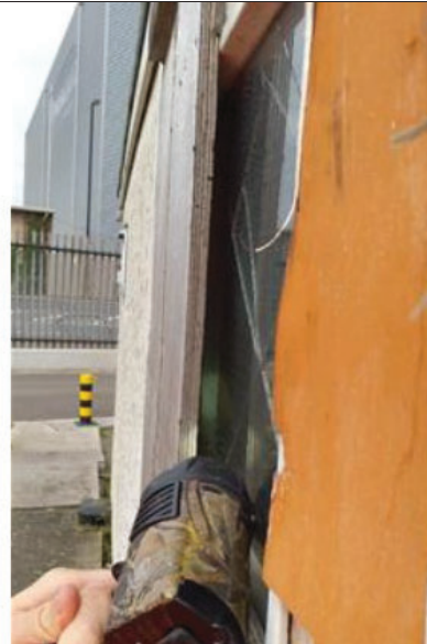
Photo 8 (24/04/2025): Building 1: boarding on broken door on south wall of extension.
