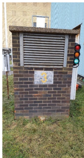
Photo 10 (24/04/2025): Structure 3, 20 m south west of Building 1 - access to underground tunnel system. Potential bat access through top of louvered vent.
