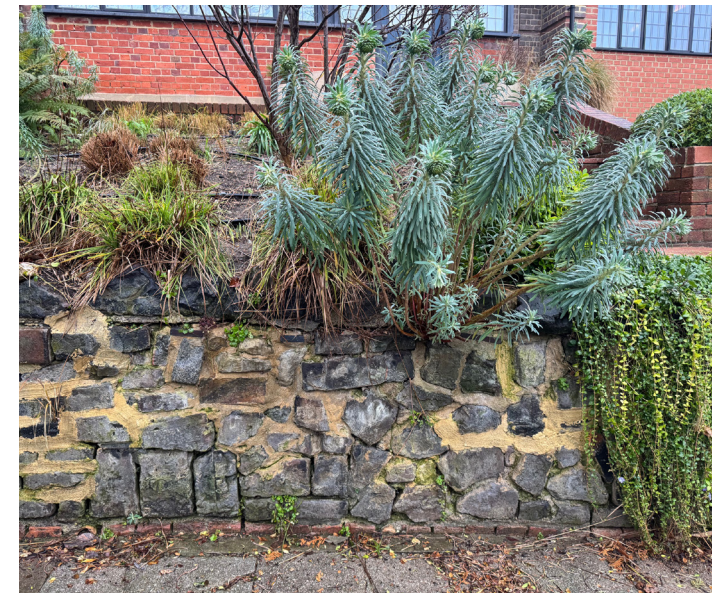
PHOTO 06 - Detailed view of front boundary wall, showing previous patch repairs, materials deterioration and evidence of water leakage
