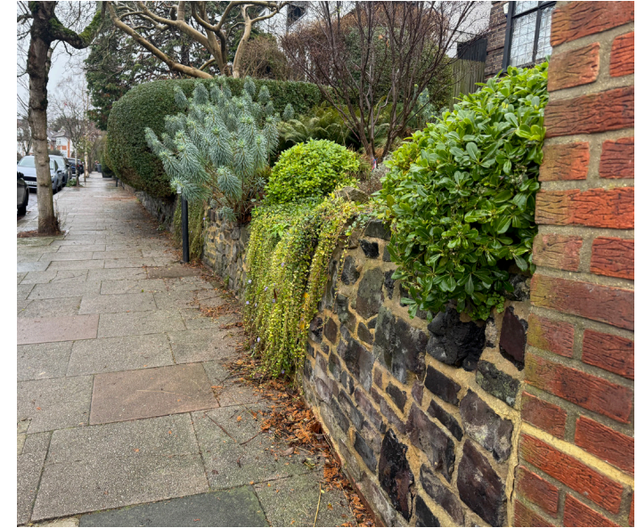
PHOTO 05 - Existing front boundary wall, showing uneven height and lack of vertical alignment
