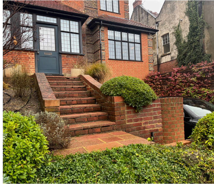
PHOTO 03 - Existing upper steps, showing narrow, steep steps with low retaining walls to either side
