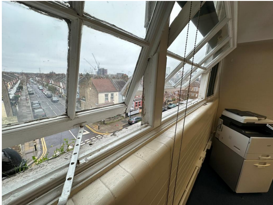
Photo showing centre pivot windows opening well past reveal.
