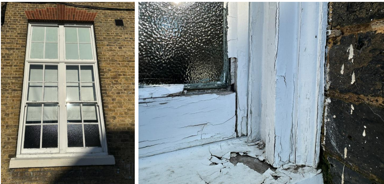
Poor condition of timber double hung sashes
