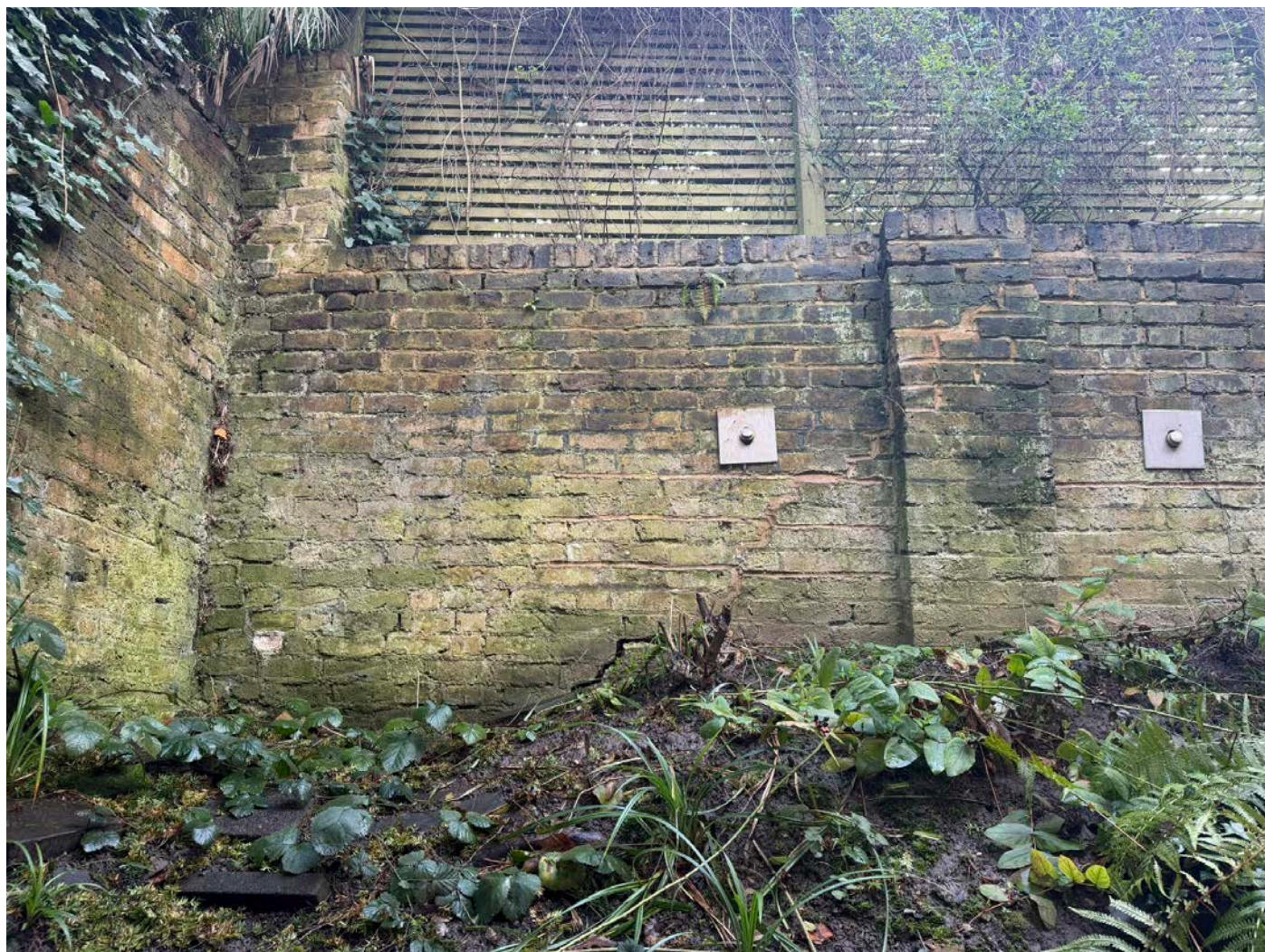
Photograph A – Uncleaned section of existing boundary wall.
