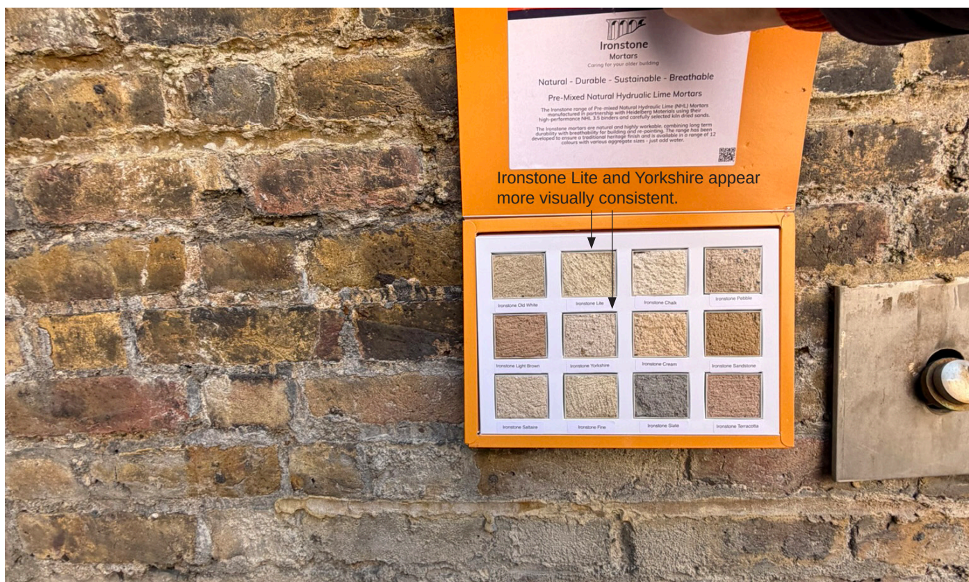
Photograph M Comparison of mortar in lower wall with example pre-mixed NHL 3.5 Lime mortars.
