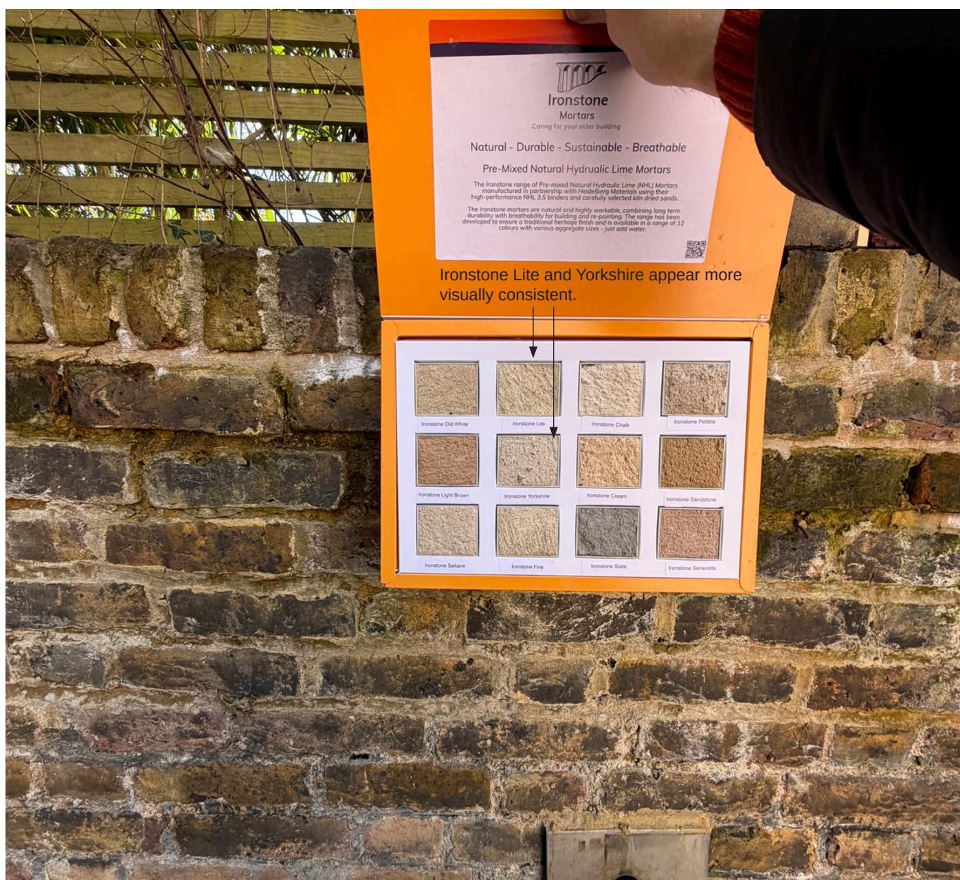
Photograph L - Comparison of mortar in upper wall with example pre-mixed NHL 3.5 Lime mortars.
