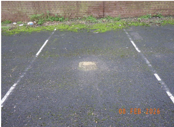
Photo 7 Location of WS02 – concreted over
