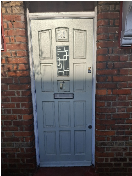
Front Entrance Door
