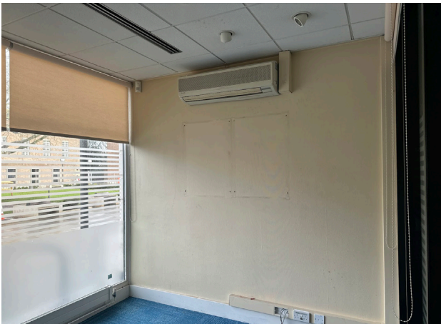
Plate 12 Room to the north east of the building showing modern services and suspended ceiling.
