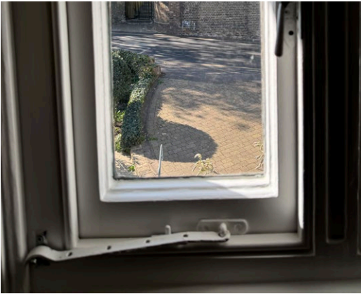
Window stay too large for casement size
