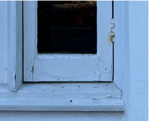
Significant splits and cracking of paintwork, woodwork rotting, white painted hinges rusting
