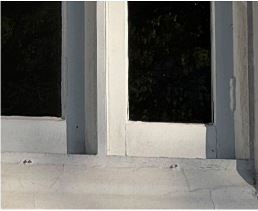
Splits in paintwork, painted over hinges and previous external latch fixings painted over
