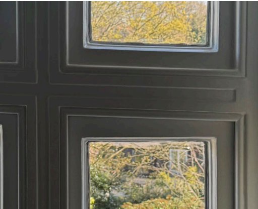
Not level transom
