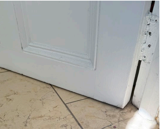
Scuff marks and chips in paintwork
