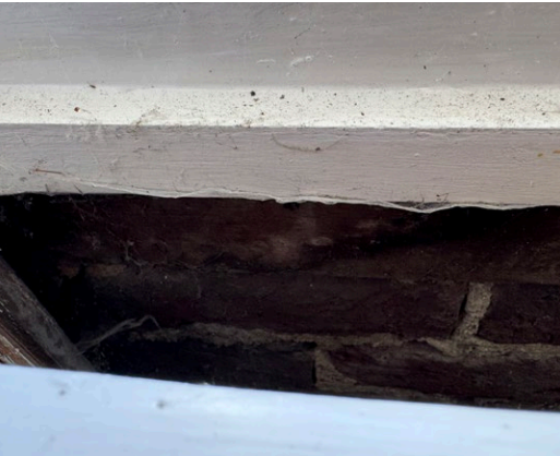
Signs of insects, weathering to paintwork
