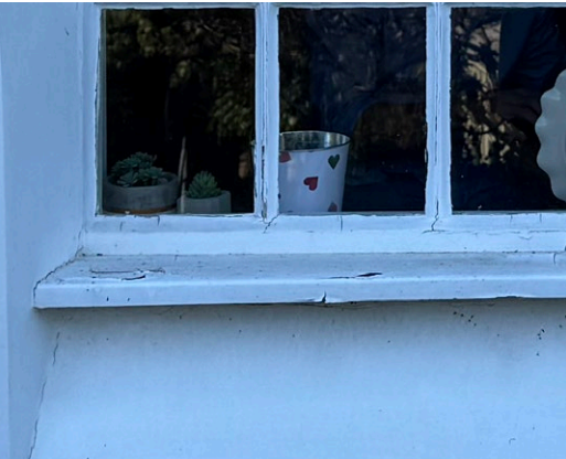
Signs of rotting on bottom rail
