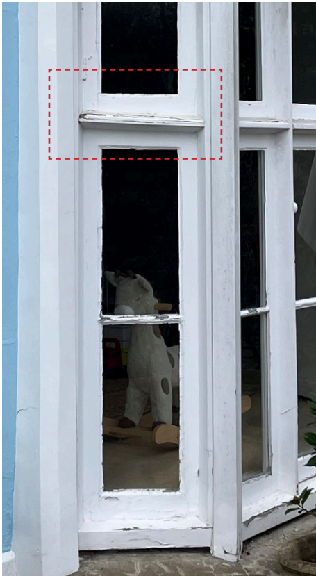
Poor external condition
