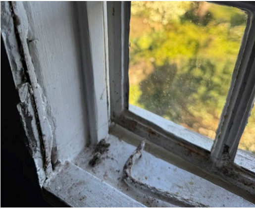
Signs of dirt, rotting and rusting of steel elements
