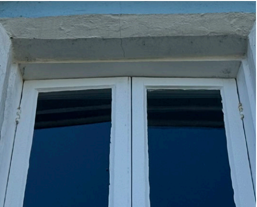
Poor airtightness-clear that window is not fully closable
