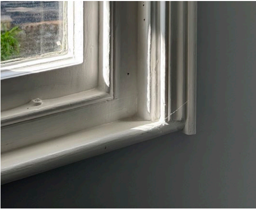
Screw marks/holes in frame
