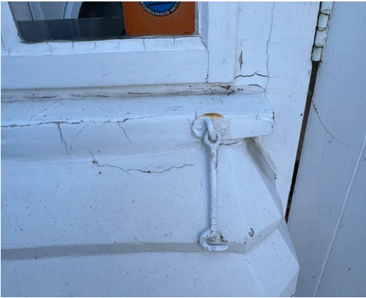
Rusting latch no longer usable alongside cracking and rotting of timber above sill
