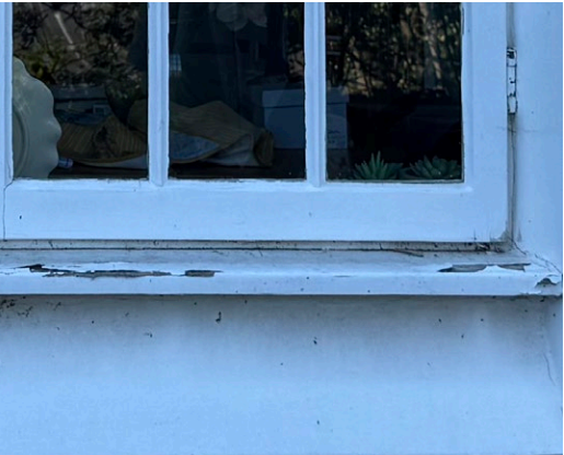
Chips and cracking in paintwork leaving exposed timber on bottom sill
