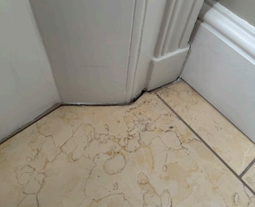
Evidence showing floor tiles covering decorative wood casing extending below floor level
