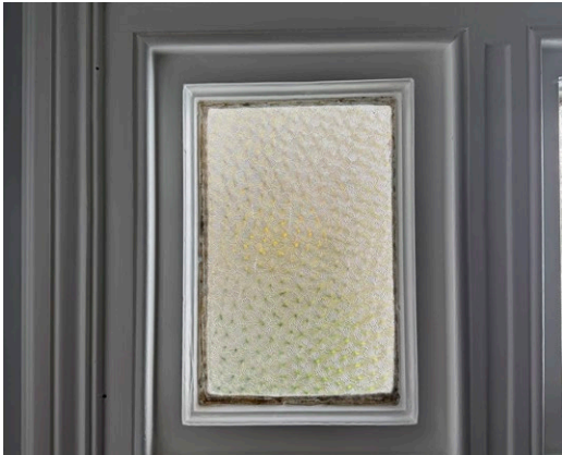
Screw/nail marks to left of glass pane, early signs of black mould along frame
