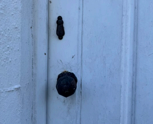
Rusting and cracking around door handle difficult to operate
