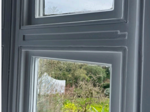
Evidence casement has been replaced - reshaped to accomodate skewed frame
