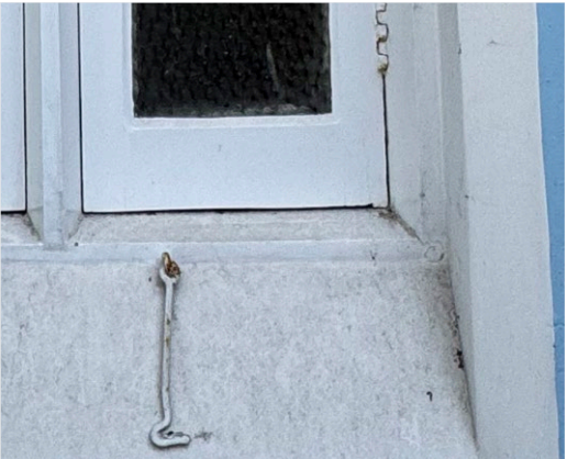
Dirt build up and weathering on decorative moulding below sill, rusting present on hinges and latches
