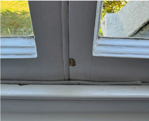
Chipped paintwork in frame, window not fully sealed when closed
