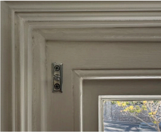
Previous fixings from blinds evident
