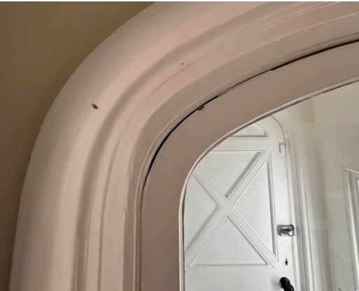
Chips in paintwork on internal frame
