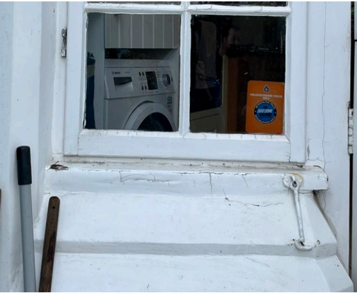
Cracks and chips in paintwork around frame and sill. Modern hinge on higher portion of stable door
