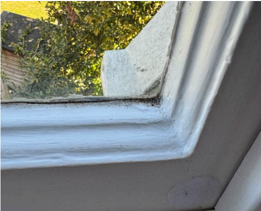
Early signs of black mould in corner of bottom rails, Velcro stickers placed in corners of frame
