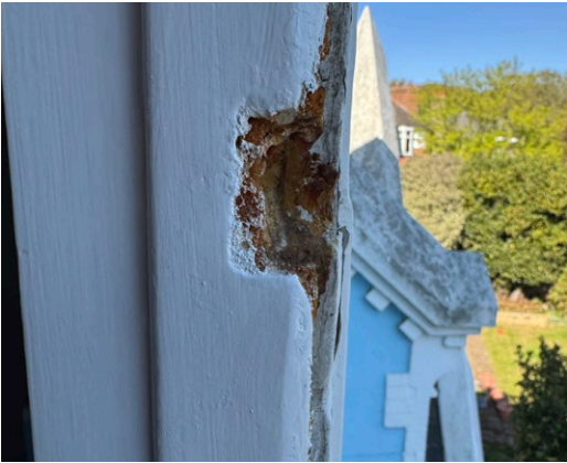
Advanced stages of rotting around lock/handle
