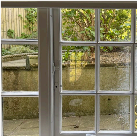
Some chips in paintwork and missing handle
