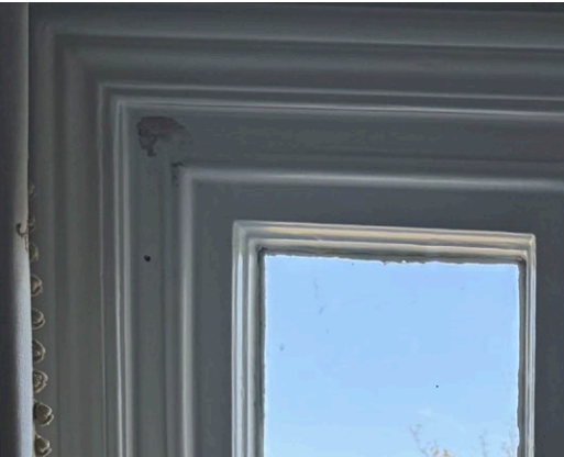
Paint flaking from frame and screw marks/holes present in frame
