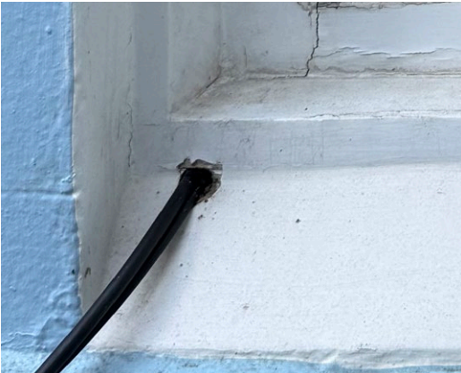
Cable entry through external plaster moulding
