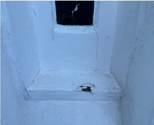
South West window: Chips and cracks in paintwork, signs of rotting in wood frame below paint
