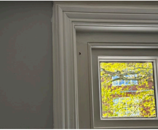
Screw marks/holes in frame
