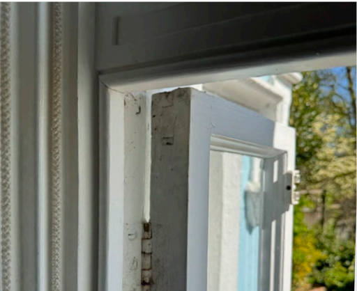
Splits in paintwork and rusting present on white painted hinges
