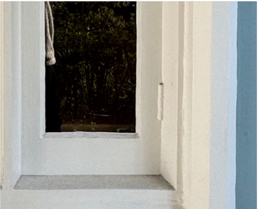
Hinges painted over to seal window casement
