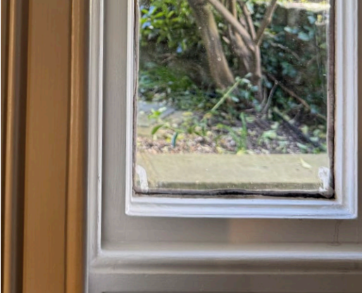
Signs of black mould on bottom rail of sills
