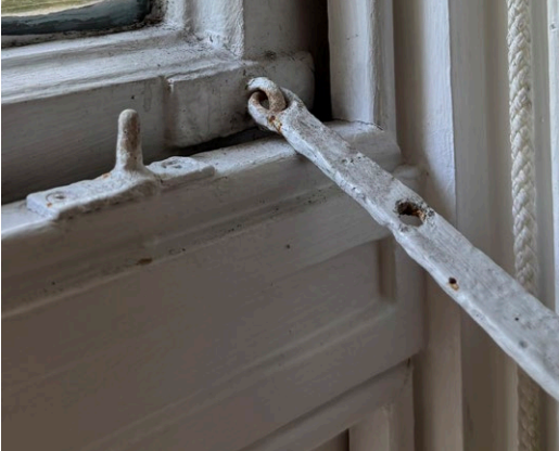
Window stay for top right casement not operable and casement not fully closable
