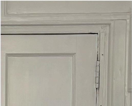
Visible gaps between door and frame
