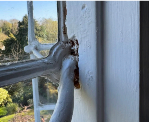
Casement not fully sealed when closed
