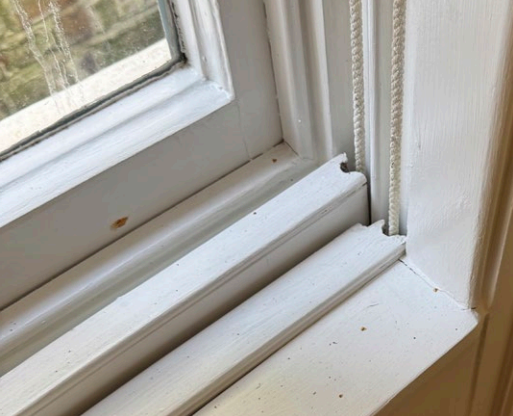
Vertical sliding shutters operable, some signs of cracking and splitting in paintwork
