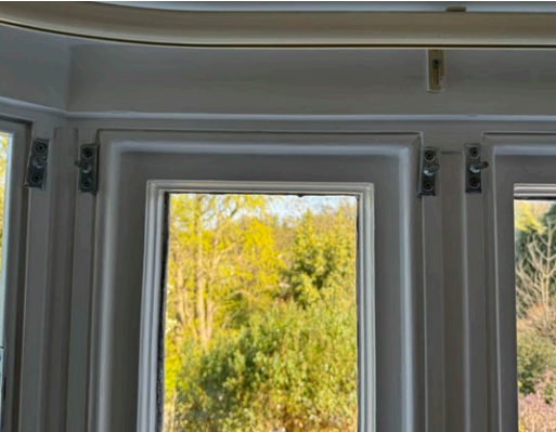
Previous blind fixings left in frame and previous curtain railed present
