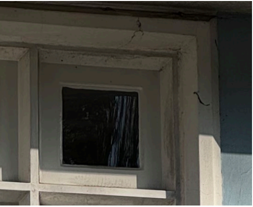
Splits and cracks in decorative moulding
