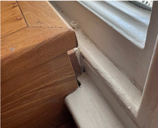
Stair overlaps and cuts into sill and frame
