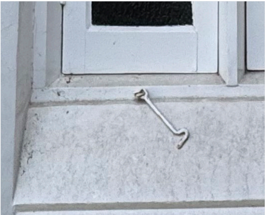
External latch and build up of dirt on decorative plaster mouldings, signs of paintwork cracking
