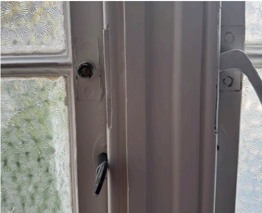
Missing handle to left casement, chips in paintwork
