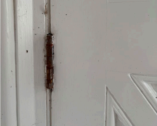
Signs of rusting on hinges and insects present around door
