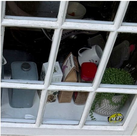
Paintwork chipped and split
