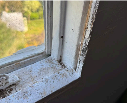
General poor condition around frame, flaking can be seen on exterior sill
