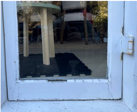
Cracks and splits in paintwork on external frames, rust on hinges
