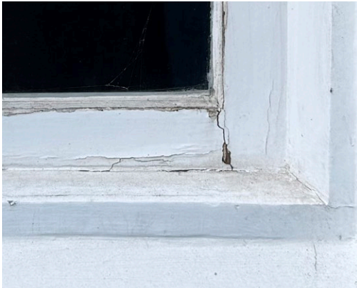
Signs of paint cracking and signs of timber rotting
