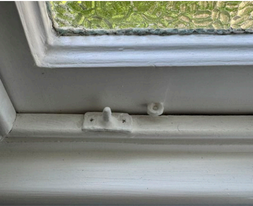
Missing window stay - window unable to be opened in fixed location
