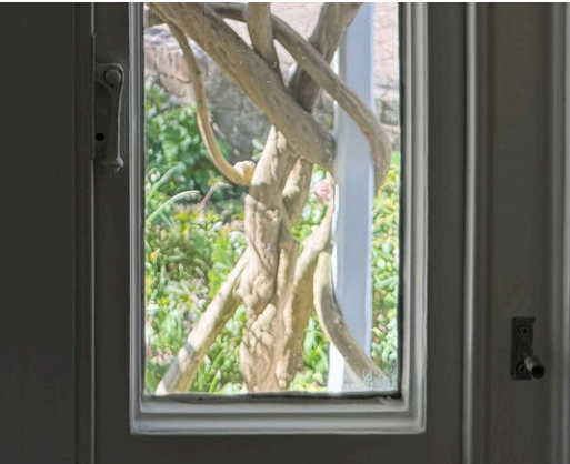
Hand and latch not fully sealing window casement
