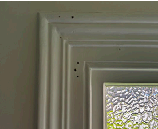
Screw marks/holes in frame and outer moulding
