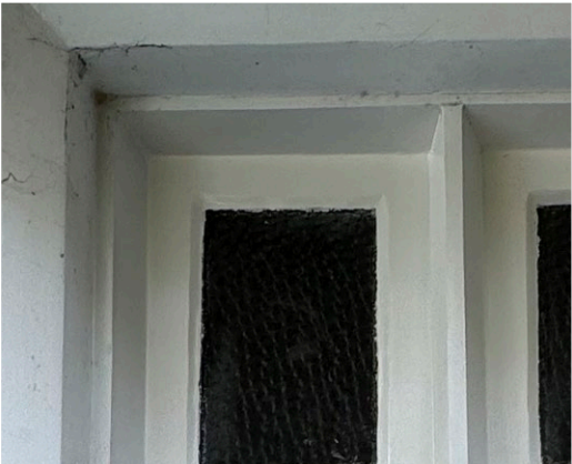
Signs of cracking and dirt build up on plaster moulding around frames
