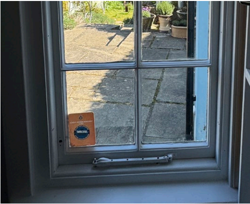
Chips in paintwork and screw/nail holes present on the frame
