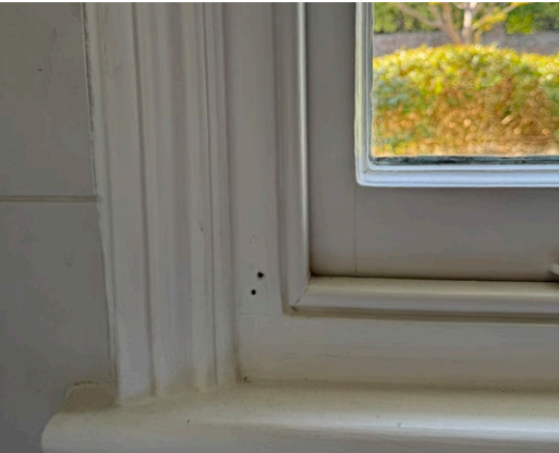
Screw holes/marks left by previous security or blind system, some splits in paintwork
