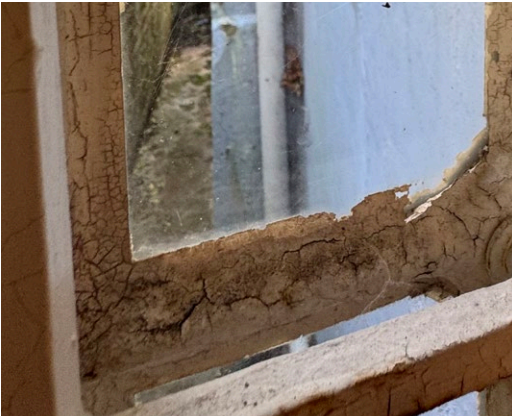
Significant signs of flaking, rotting and rusting
