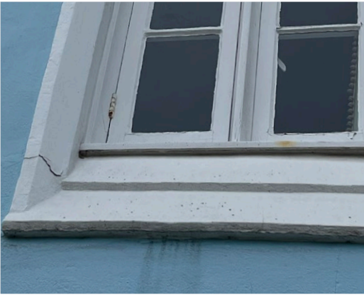
Cill in poor condition
