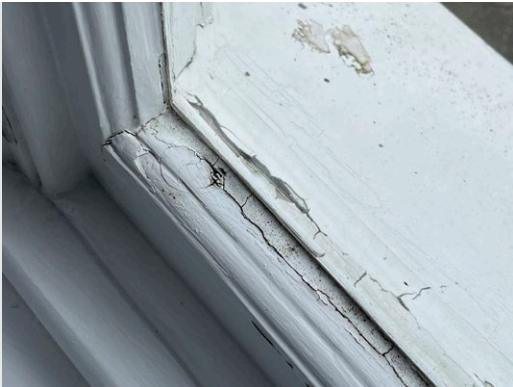
Evidence of cracking and rotting in timber frames
