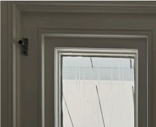
Previous blind fixings left in frame
