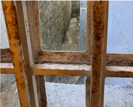
Significant sign of rusting, cracking and rotting
