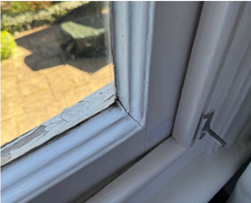
Splits and cracks in woodwork -condition of external sill is visible
