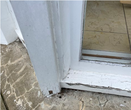
Damage to post and cill
