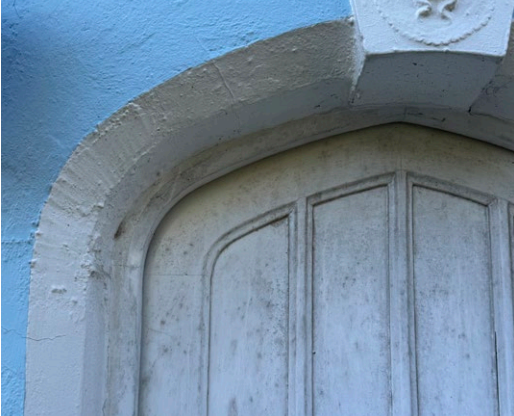
Signs of weathering on top portion of door
