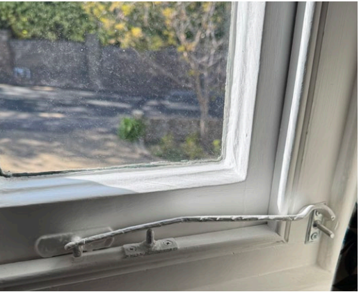
Window stay too large for casement size and poorly painted
