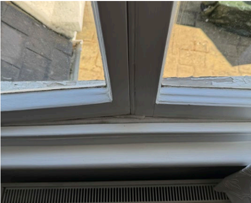
Significant gaps to exterior. Large brush seal placed around frame to reduce draft
