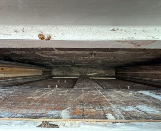
15cm discrepancy between bottom of timber shutter casing and floor level -rubble present at base.
