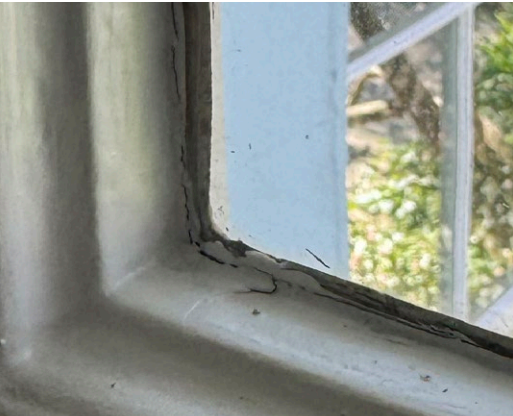
Early signs of rotting and splitting directly around glass pane
