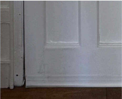
Scuff along bottom rail
