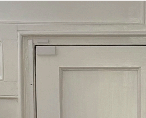
Security systems in place
