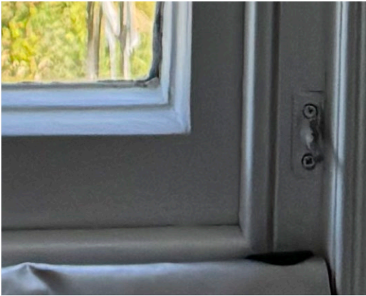
Previous blind fixings left in frame
