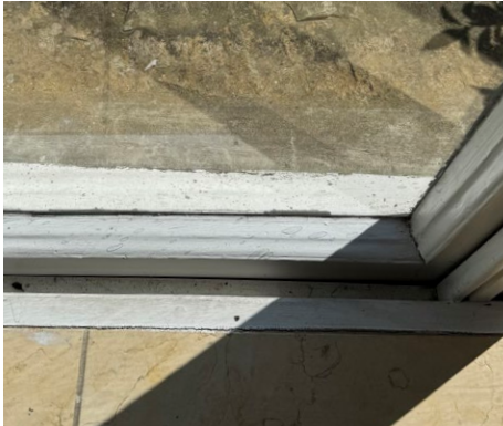
Window sill finished below floor level
