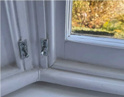
Previous blind fixings left in frame and evidence of cracking and rotting in timber frames
