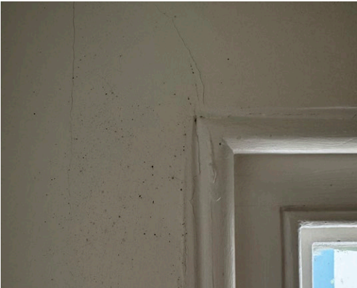
South West Window: Black mould around interior decorative moulding
