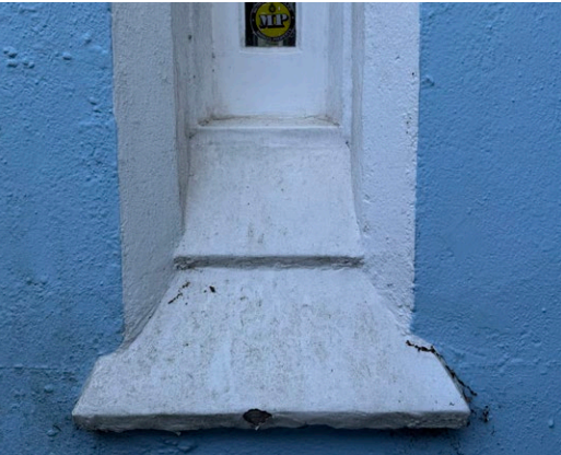
North East Window: Signs of weathering on decorative moulding around window
