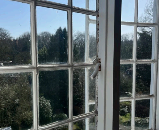
Advanced rotting and signs of black mould on rails
