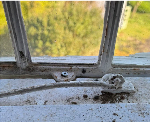
Build up of dirt, black mould and rusting, evidence of ladybirds and fixing screwed shut
