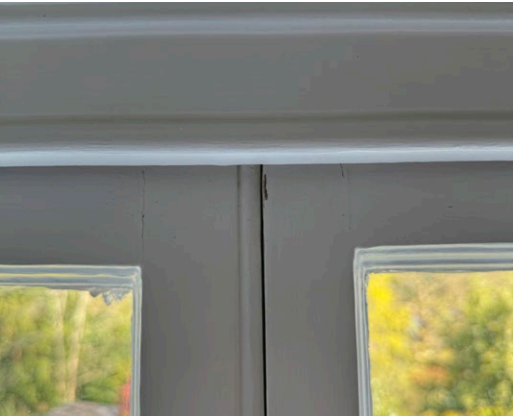
Splitting and chips in wood/paint work
