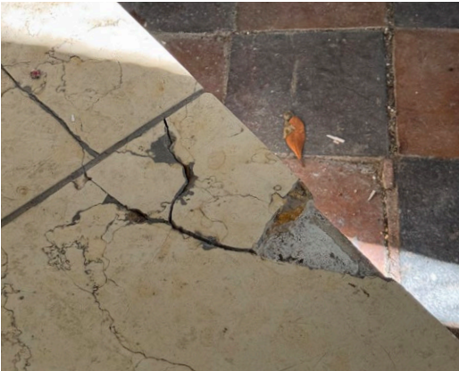
Tiles cracked and chipped away in door opening
