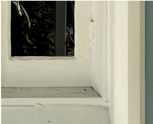
Hinges on previously operable casement painted over and sealed
