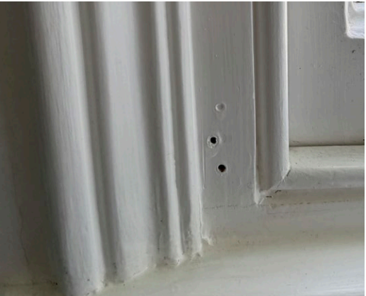
Screw marks/holes in frame
