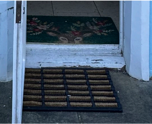
Significant scuff marks, chips and cracking to threshold timber on door
