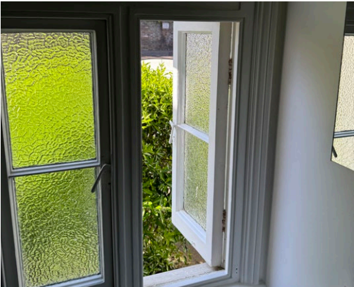
Window unable to be opened in fixed location
