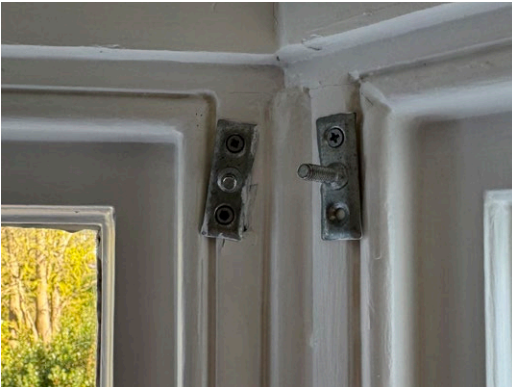
Previous blind fixings left in frame
