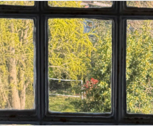
Broken window pane with hole to exterior
