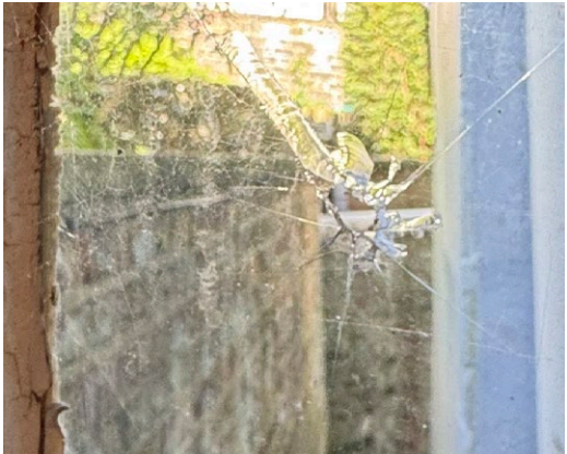
Crack and hole evident in one glass pane
