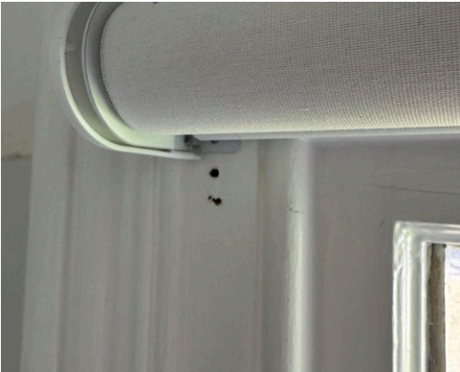
Screw holes/marks left by previous security or blind system
