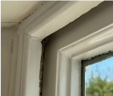
Casement not fully closable
