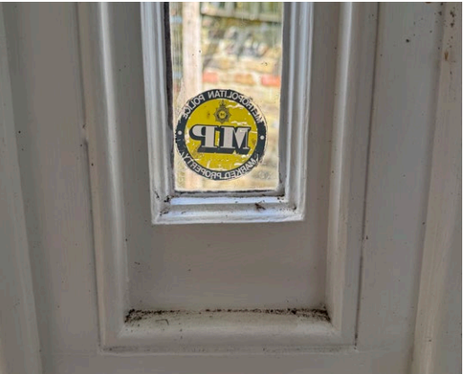
North East Window: dirt, insects and cobwebs on sill, manufacturer sticker on glass
