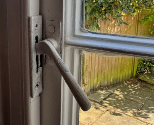
Steel handle painted over poorly with chips and flaking of paintwork
