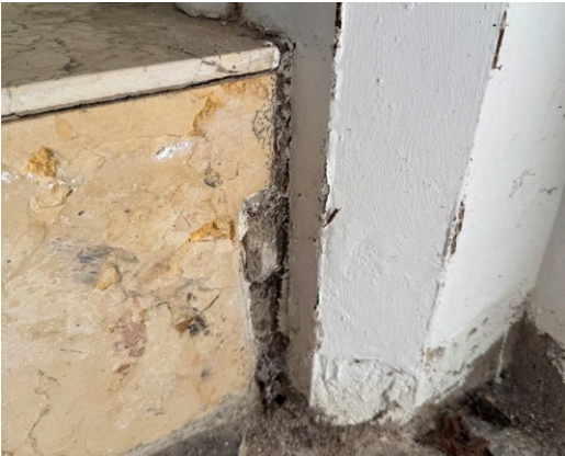
Signs of rotting on inner post (jamb)
