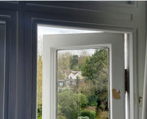
Evidence casement has been replaced to fit within skewed transom
