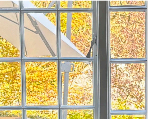
Evidence of insects on woodwork
