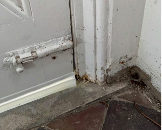
Signs of rotting where door frame meets ground, paintwork flaking and chipped
