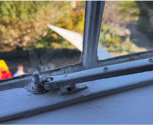
Holes in window stays painted over therefore not fully operable.
