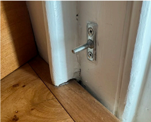
Previous blind or security fixings left in frame
