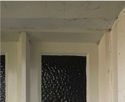
Signs of cobwebs, splitting and cracking of paintwork around frame
