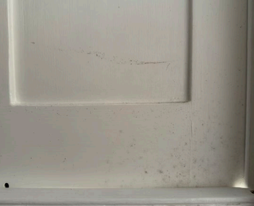
Vertical sliding shutters operable with signs of mould on timber panels
