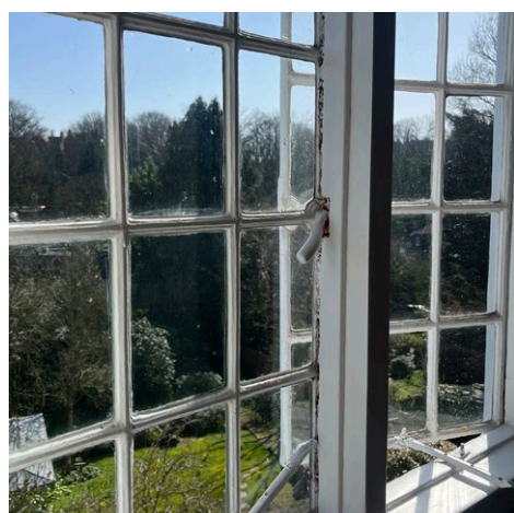
WFF.03 (REAR) First Floor Bedroom Very poor condition
