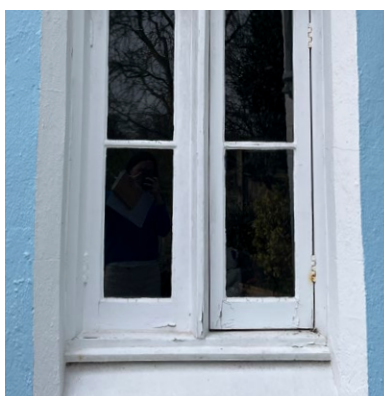
WLG.010 (REAR) Lower Ground Floor Living Room Poor external condition
