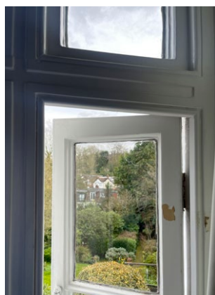
Casement has been replaced to fit within distorted opening
