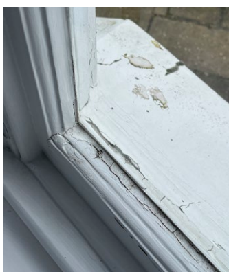
WUG.10 (REAR) Upper Ground Floor Bay Window Poor external condition
