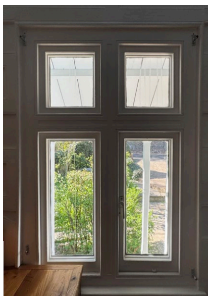
WUG.03 (FRONT) Upper Ground Floor Stair Previous fixings left behind
