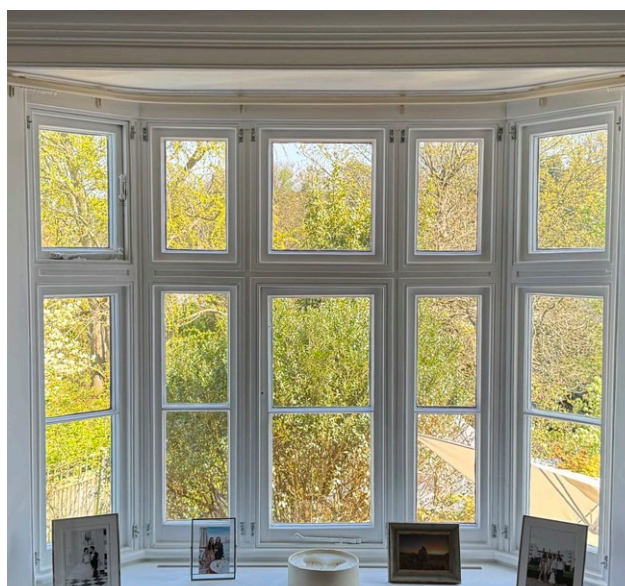
WUG.10 (REAR) Upper Ground Floor Bay Window Previous fixings left behind
