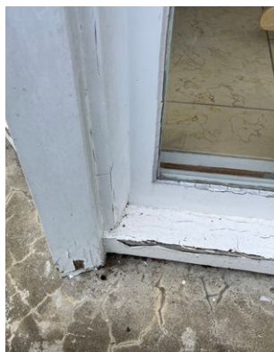
WLG.011 (REAR) Lower Ground Floor Bay Window Structural post is splitting and rotting
