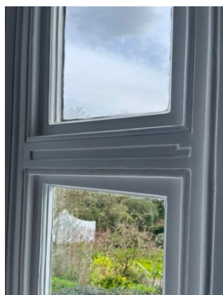
WUG.10 (REAR) Upper Ground Floor Bay Window Transom not level and replacement casement
