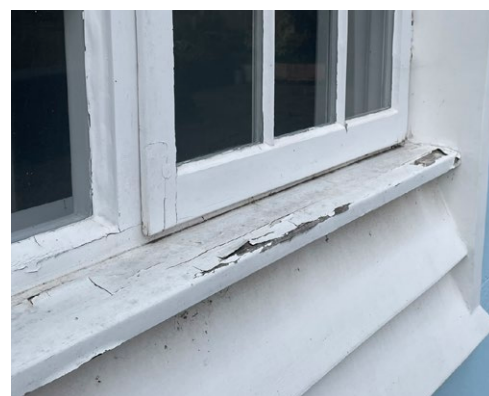
WUG.08 (REAR) Kitchen Window Poor external condition
