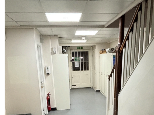
Fig. 10 Escape door proposed for replacement
