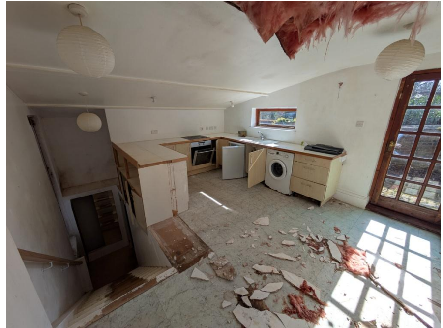
Upper kitchen level in derelict condition with roof collapse.
