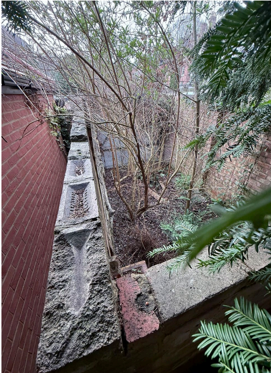
Existing walls, decayed roof and vegetation at boundary with neighbouring garage
