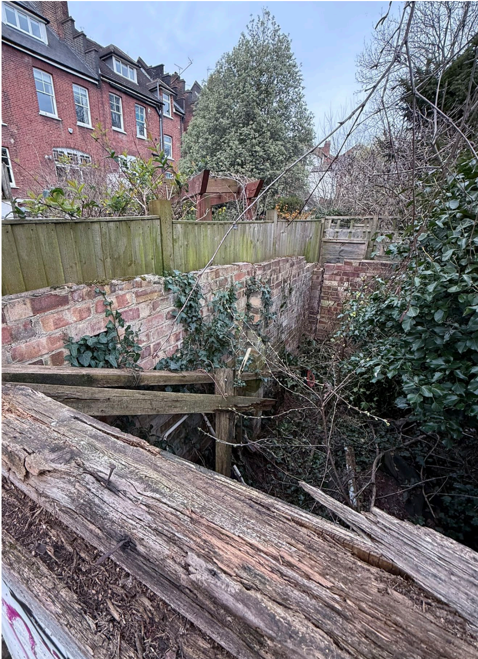
Existing walls, decayed roof and vegetation at boundary with 8 Coolhurst Road
