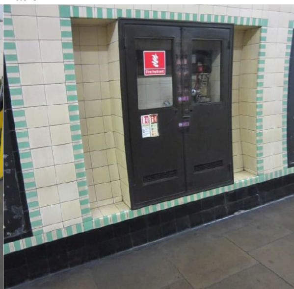
Photo 4.15: Original fire hydrant cabinet on Platform 1
