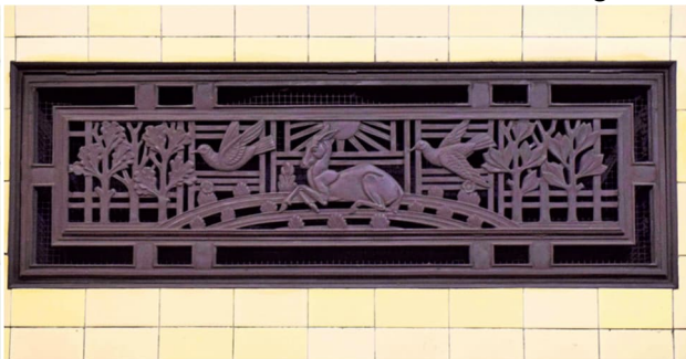
Photo 4.12: Decorative bronze ventilation grilles
