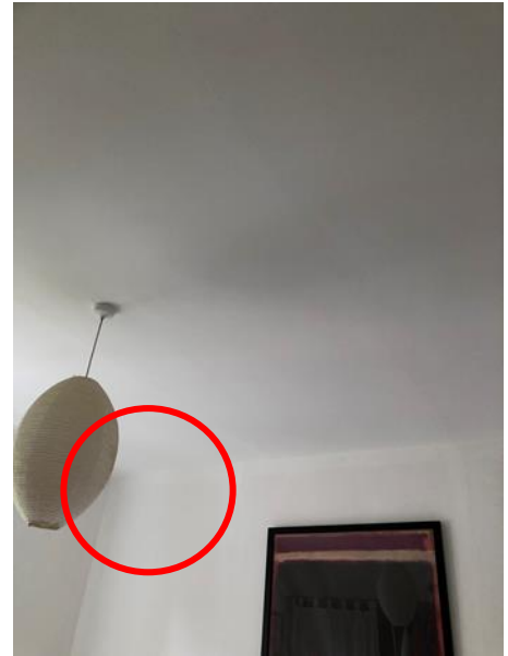
Photo 26: Area of vertical and diagonal hairline and fine cracks to flank wall
