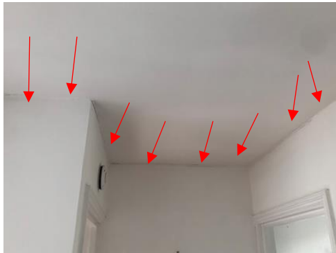
Photo 48: Fine cracking throughout
