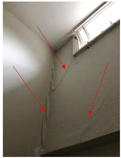
Photo 59: Closer view of diagonal cracks beneath paper and rippling to wallpaper
