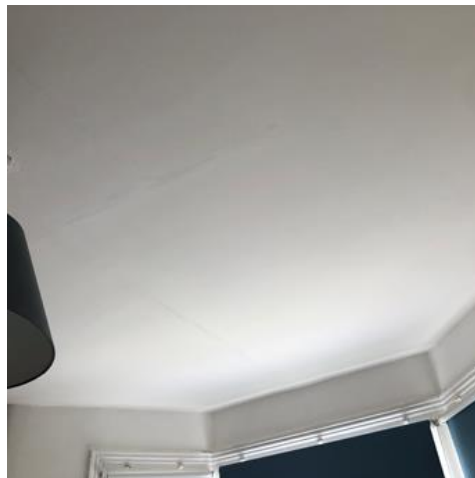
Photo 30: General cracks to ceiling throughout
