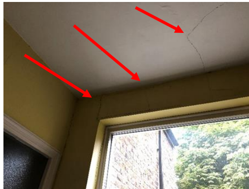
Photo 21: Close up view of cracks
