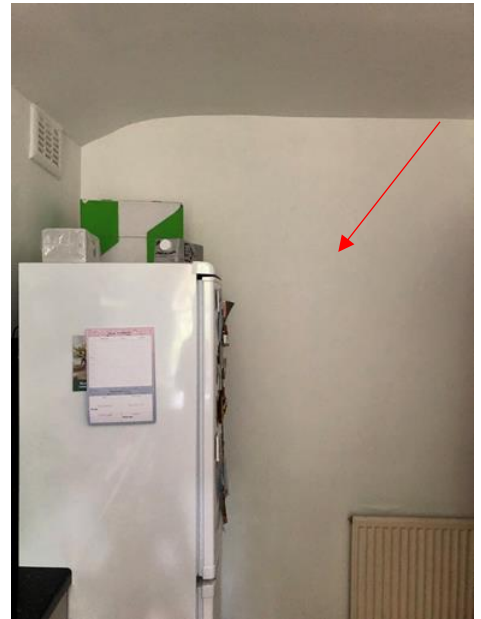
Photo 37: Minor vertical hairline crack to partition with communal area
