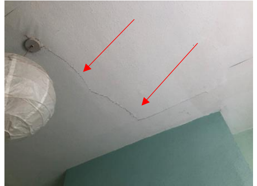
Photo 14: Fine cracks to ceiling
