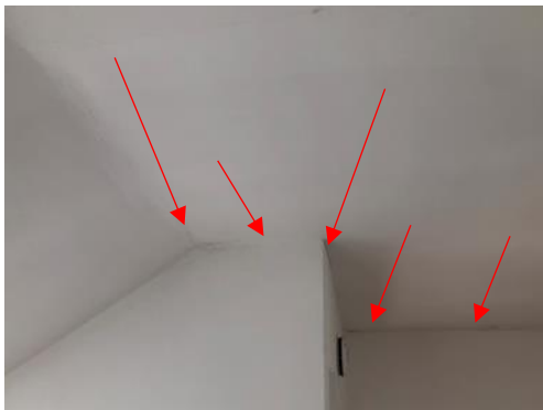
Photo 47: Fine cracking to junction of ceiling/walls throughout stairs, half landing and landing
