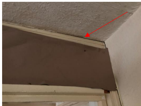
Photo 19: Separation cracks above door
