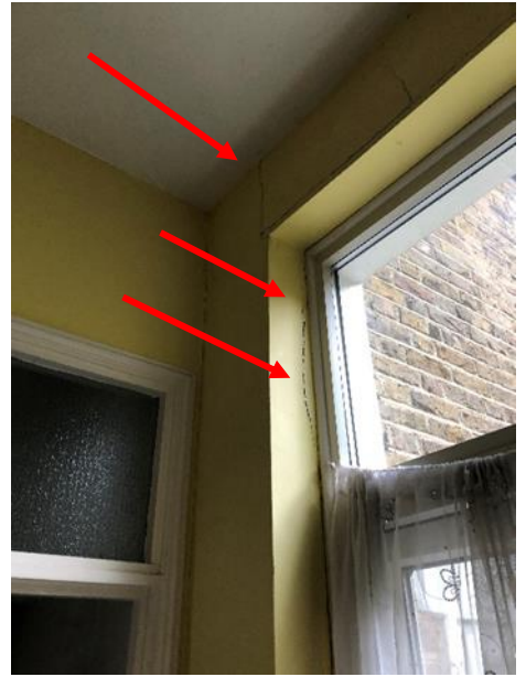
Photo 20: Vertical fine cracks above door & surround to garden
