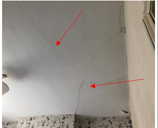
Photo 12: Crazed fine cracks to ceiling / rear of room
