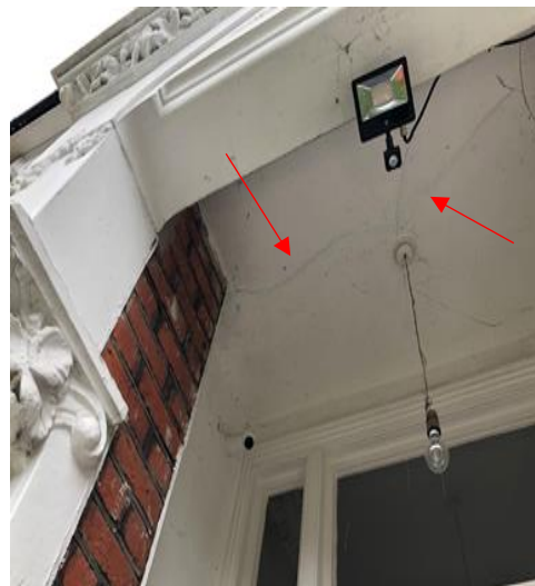
Photo 62: Porch ceiling – crazed cracking
