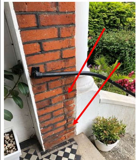
Photo 63: Stepped cracks to brickwork
