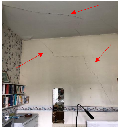
Photo 11: Diagonal fine cracks to partition with bedroom 2
