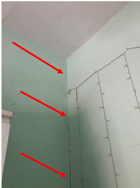
Photo 15: Fine vertical cracks to rear wall / partition with front bedroom
