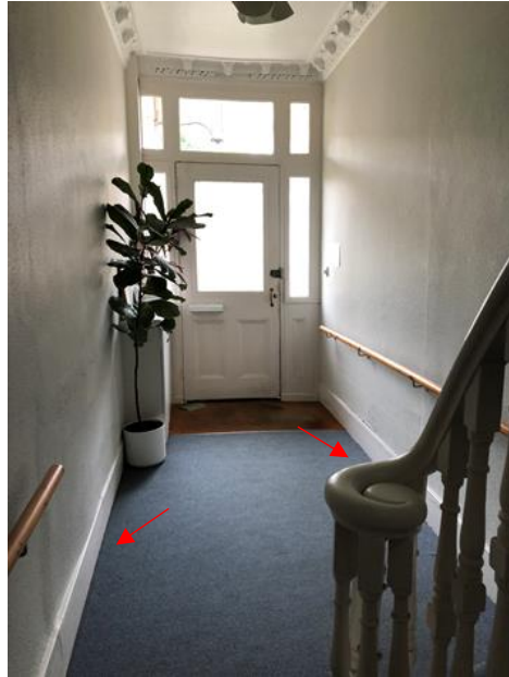
Photo 56: Overview of communal entrance, sloping flooring as shown by arrows
