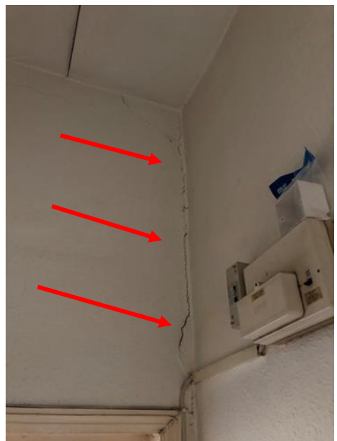
Photo 8: Vertical cracks above entrance to living room
