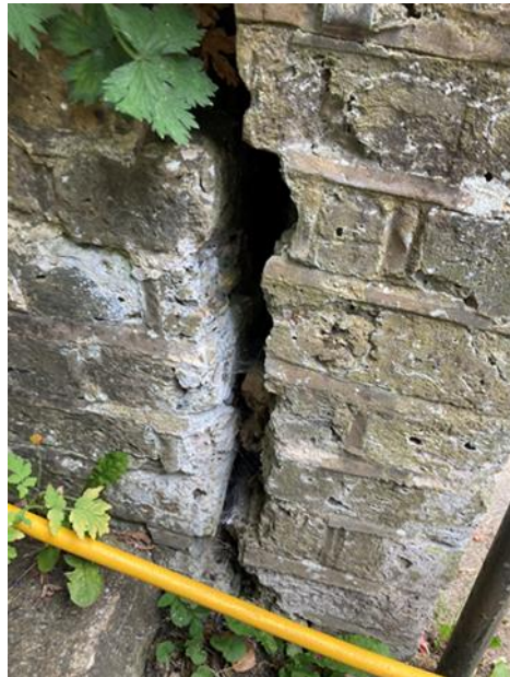
Photo 74: Opened up crack to garden wall - Area 1
