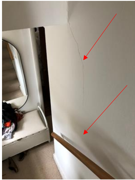
Photo 34: Closer view of fine vertical crack
