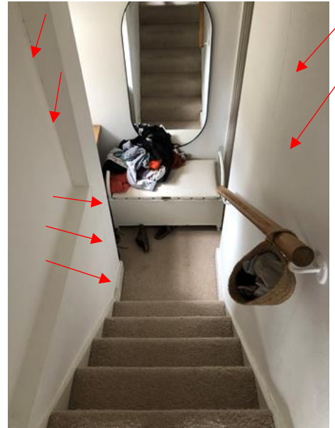
Photo 33: Overview of stairs leading to bathroom and kitchen to rear. Fine cracks to both sides of stairwell
