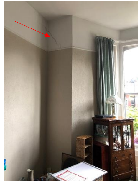
Photo 21: Close up view of fine diagonal and horizontal cracking / left hand side of bay window
