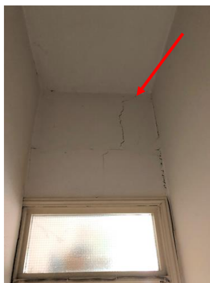
Photo 4: Fine vertical cracks above entrance to front bedroom
