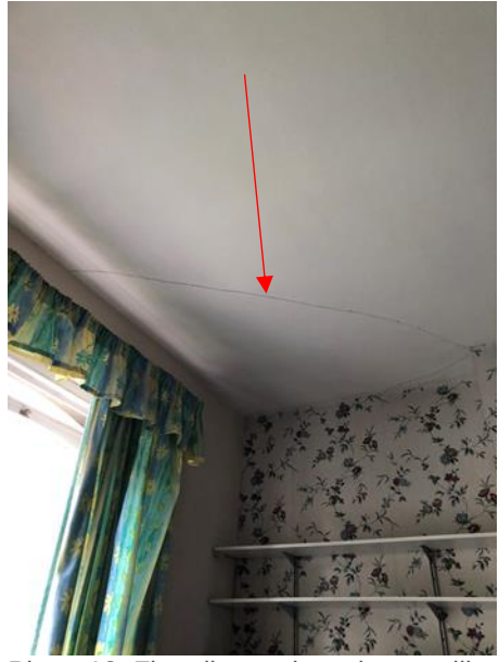
Photo 10: Fine diagonal cracks to ceiling / front elevation
