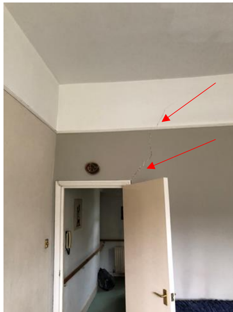
Photo 22: Fine diagonal crack above entrance door
