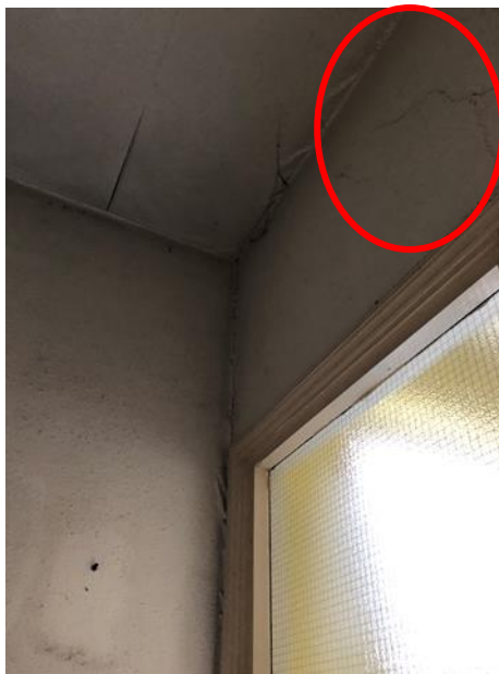
Photo 7: Fine diagonal cracks above entrance to kitchen
