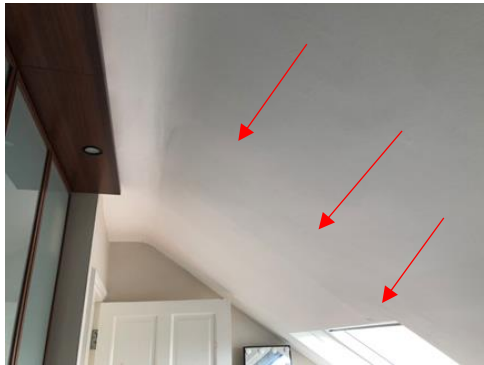
Photo 50: Overview of ceiling with general hairline cracks to boards
