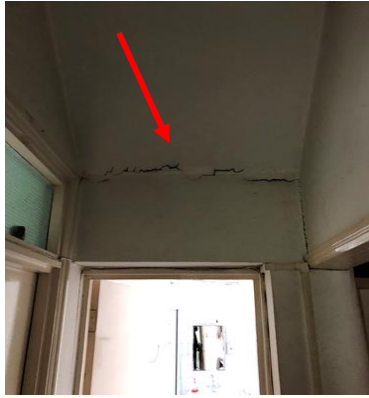
Photo 5: Horizontal cracking across top of entrance to rear bathroom
