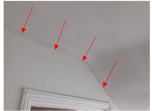
Photo 49: Close view of fine horizontal cracks above door to living room
