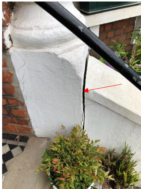
Photo 64: Gap to top top of stairs
