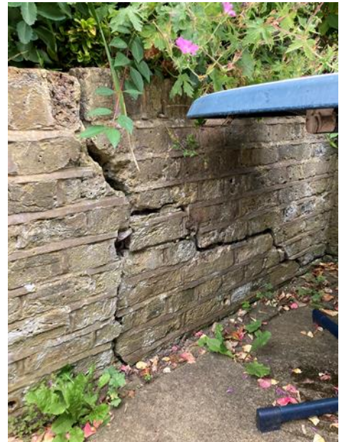
Photo 75: Stepped opened up cracking to garden wall – Area 2
