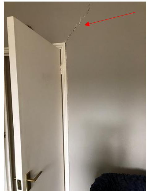
Photo 23: Close up view of diagonal crack above entrance door
