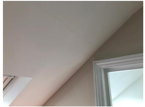
Photo 55: Fine cracks to ceiling plasterboard
