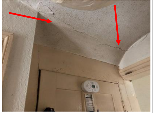
Photo 6: Fine horizontal cracks above entrance to Cellar
