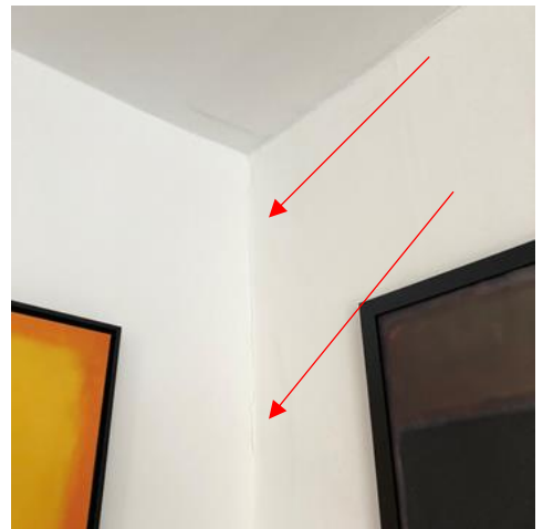
Photo 31: Hairline cracks to corner of partition wall with bathroom/flank wall
