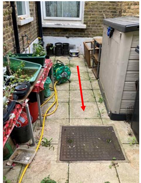
Photo 79: Rear patio area – floor slanting
