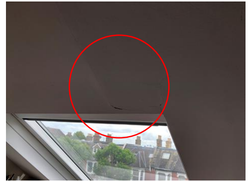
Photo 51: Closer view of hairline cracks above window, opposite entrance door
