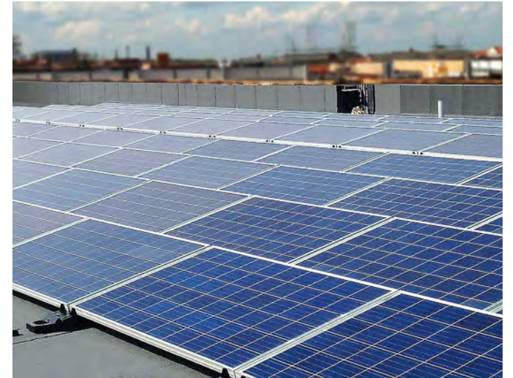
Solar PV Panels
