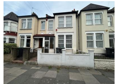
Fig. 3 — Front elevation of No. 22, with later cement render obscuring the original brickwork.
