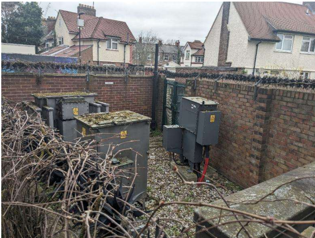
PHOTOGRAPH 2: ELECTRICITY SUBSTATION IN NORTHWEST OF SITE
