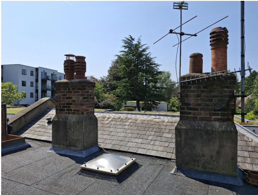
Figure 8 The existing chimneys are now much altered and have lost the characteristic "zig zag shape" noted in Plate 3
