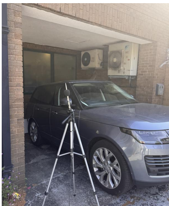
Figure 4.1 Measurement of Topps Tiles condenser units
