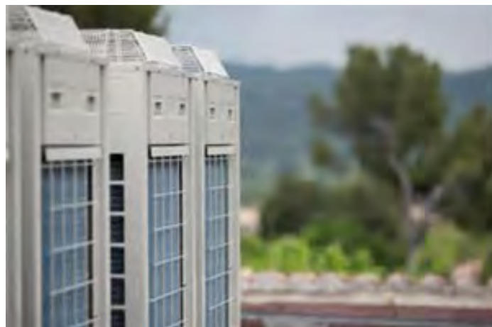
Typical ASHP Outdoor Units
