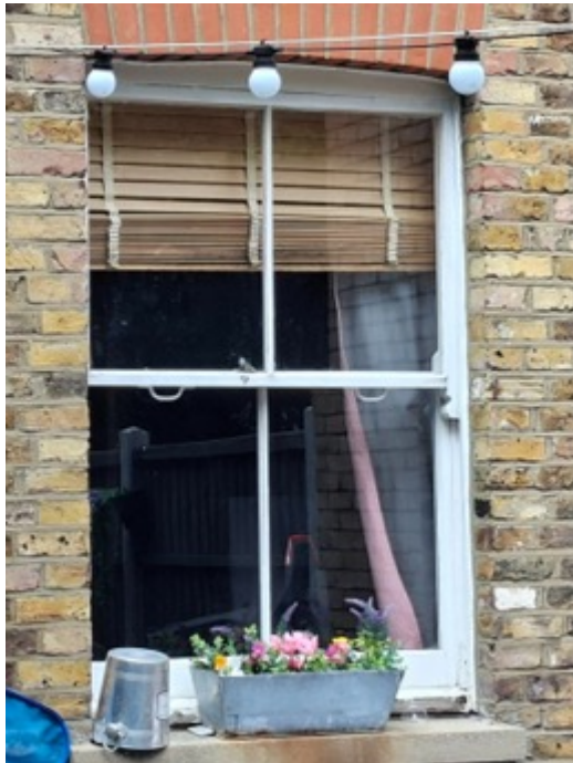
Rear End Ground Floor Window
