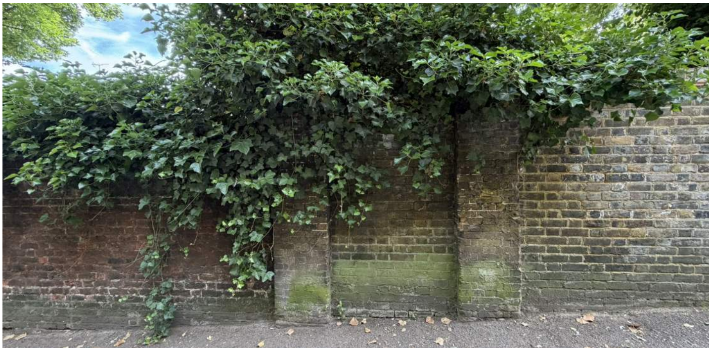
Photograph C - Showing detailing of two pillars within the wall and extensive planted overgrowth. There is no grey/blue plinth stone within the wall at this location or at its base.
