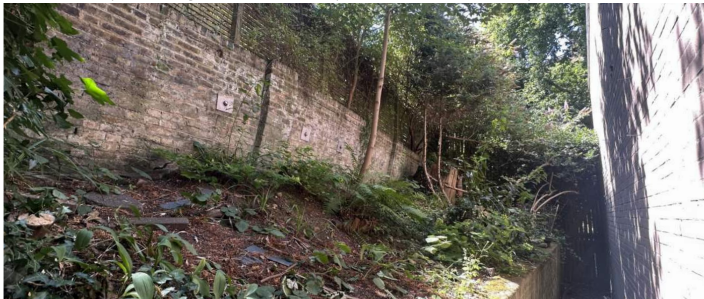
Photograph S - Photograph showing failing boundary wall between no. 84/Highstone House and no.86, not visible from the public realm.
