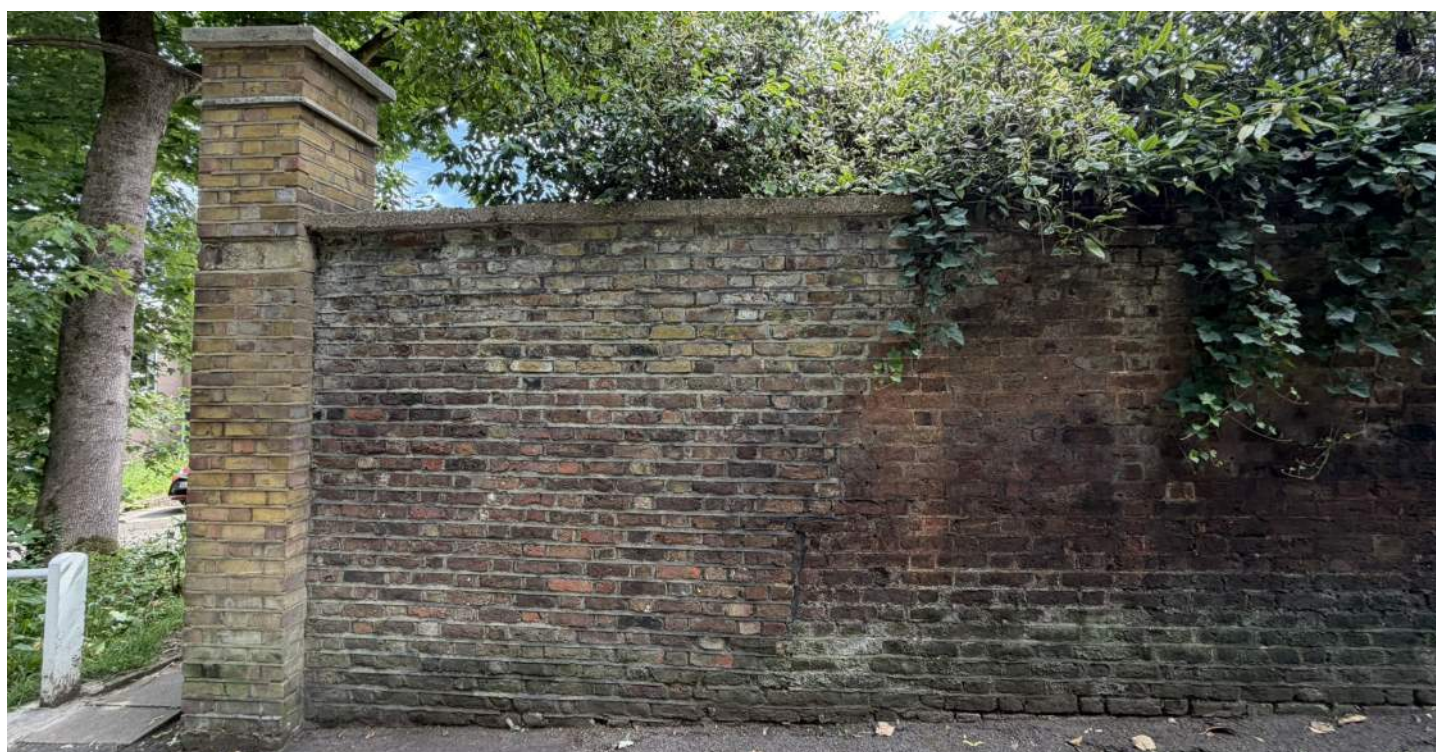
Photograph B - Showing the Boundary wall next to the pillar having a uniform brick appearance with a solid grey coping stone on the top of the wall. There is no grey/blue plinth stone within the wall or at its base.
