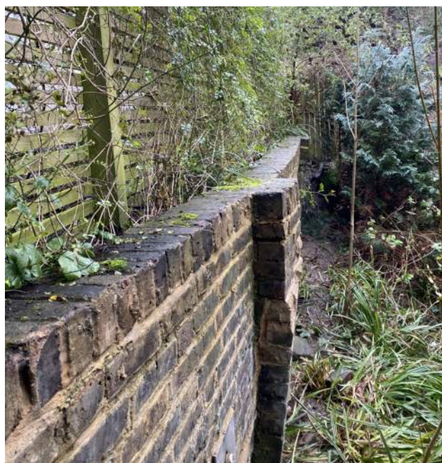
Photograph T - showing the poor condition of buttressing with a flat top and brick header courses as modified by application HGY/2014/3447
