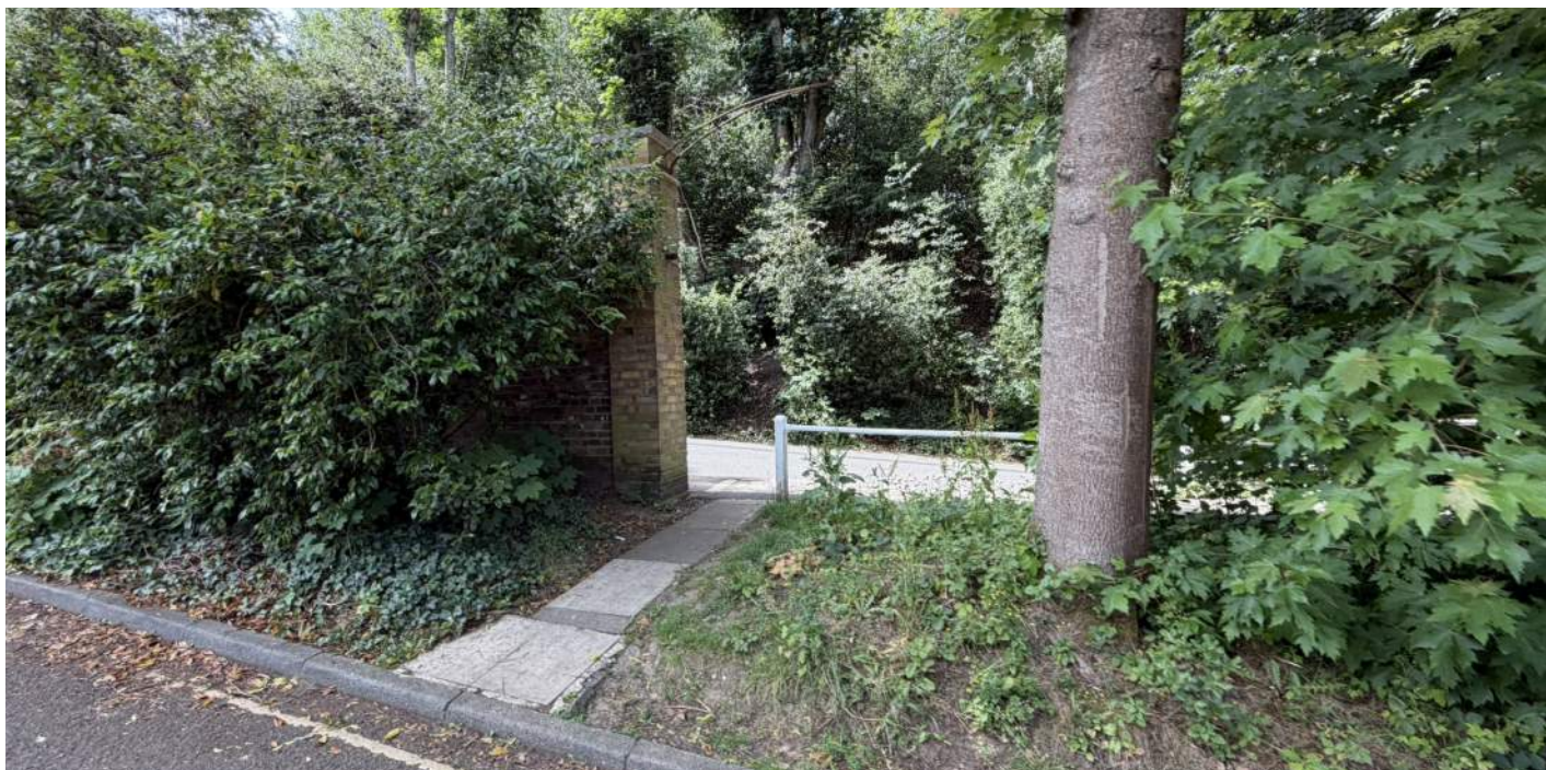
Photograph H - Showing the end condition of the wall connecting to the public highway (the opposite side of Photograph B). There are no blue/grey plinth stones at this location.
