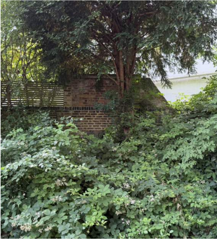
Photograph Q - Shows the contrasted difference between the lower weathered yellow stock bricks with a vertical header course and an upper diagonally climbing course of primarily red bricks which presumably was a later addition made to the wall which caps off a boiler room to no 84/Highstone House behind it.
