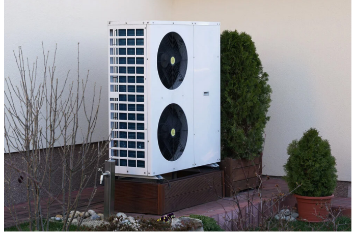
Air-source heat pump.
