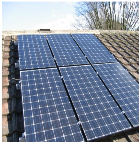
Figure 4 - Photovoltaic array on a pitched roof
