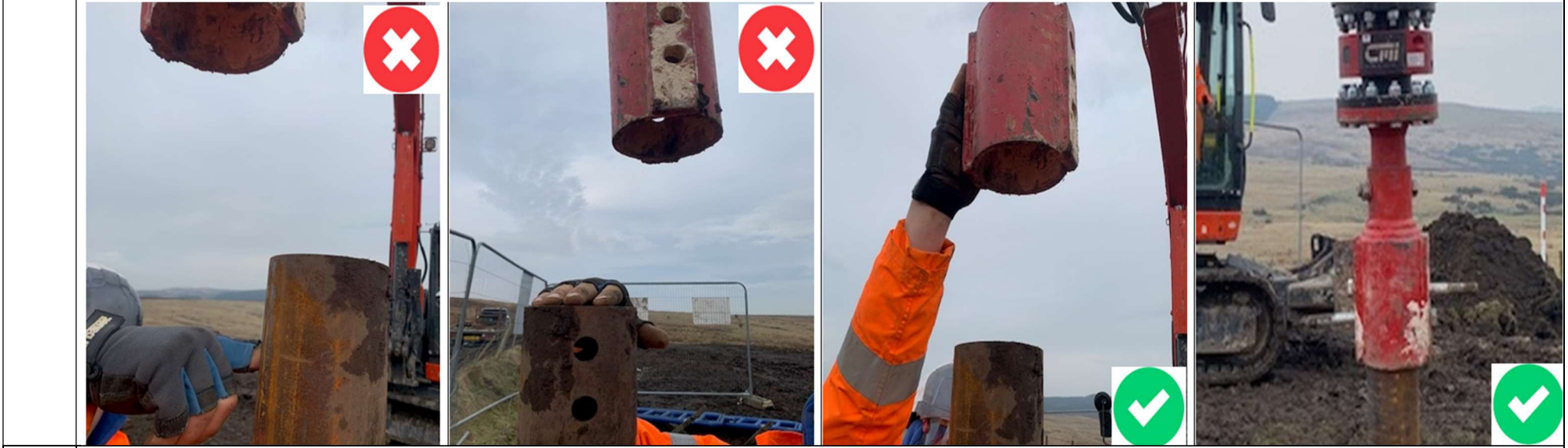
10 Personnel Protective Equipment
