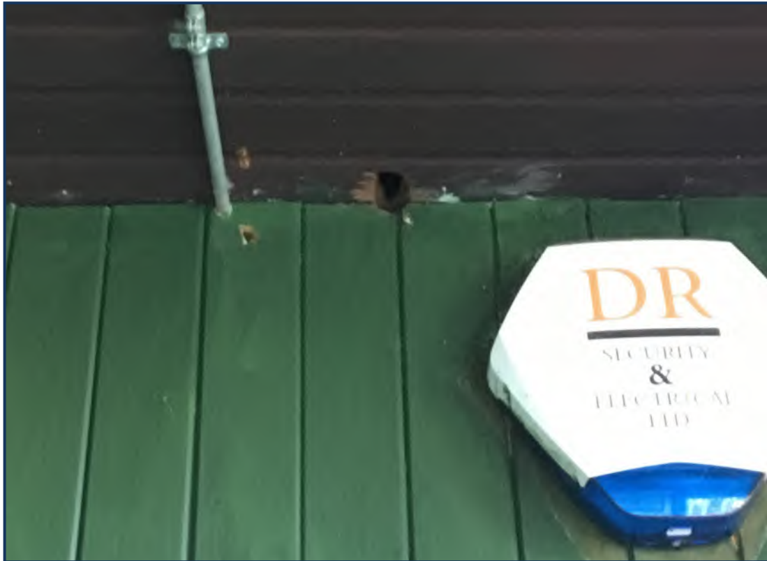
PHOTOGRAPH 9: Building B1 - Gap in Wood
