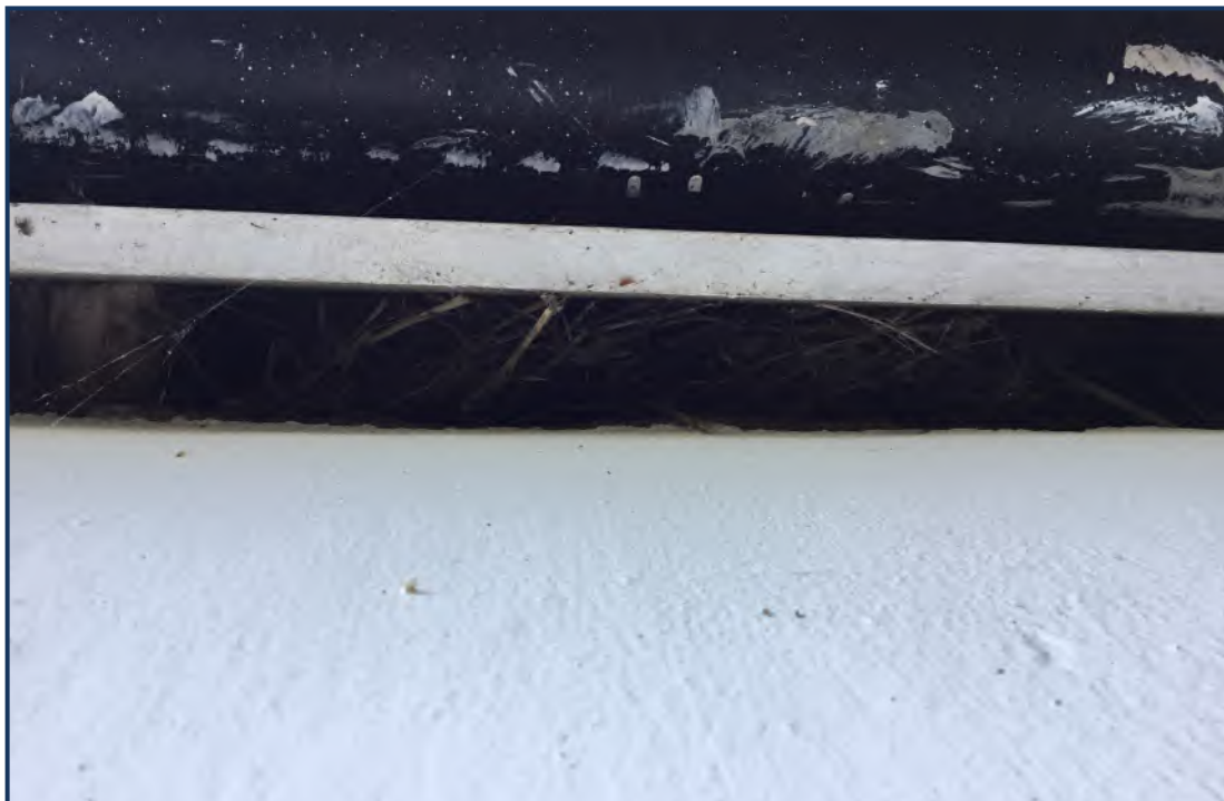
PHOTOGRAPH 6: Building B1 - Gap in Barge Board
