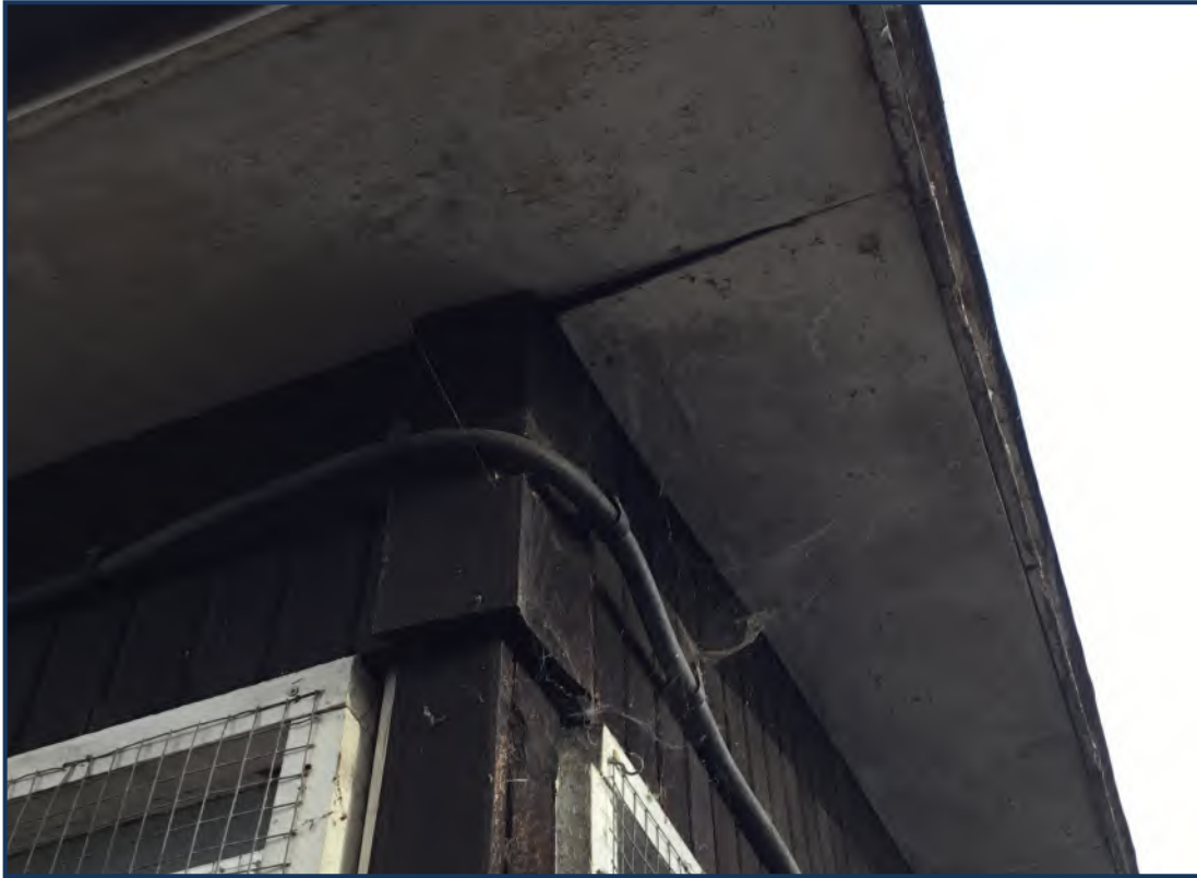
PHOTOGRAPH 7: Building B1 - Gap in Soffit Board
