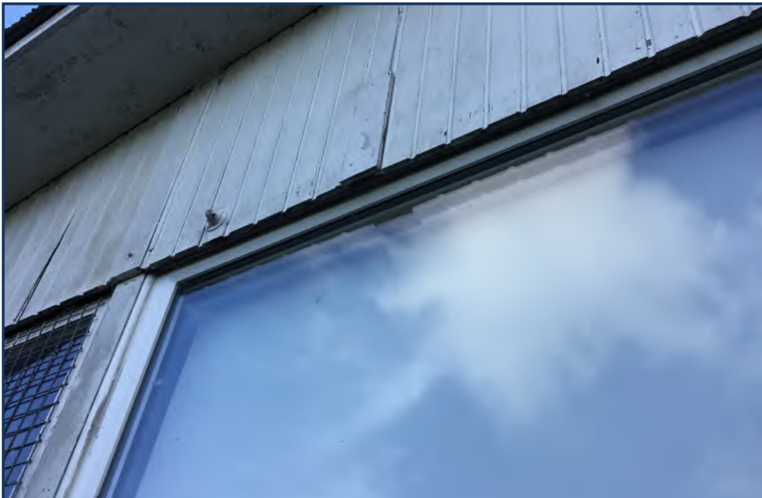
PHOTOGRAPH 8: Building B1 - Gaps in Cladding
