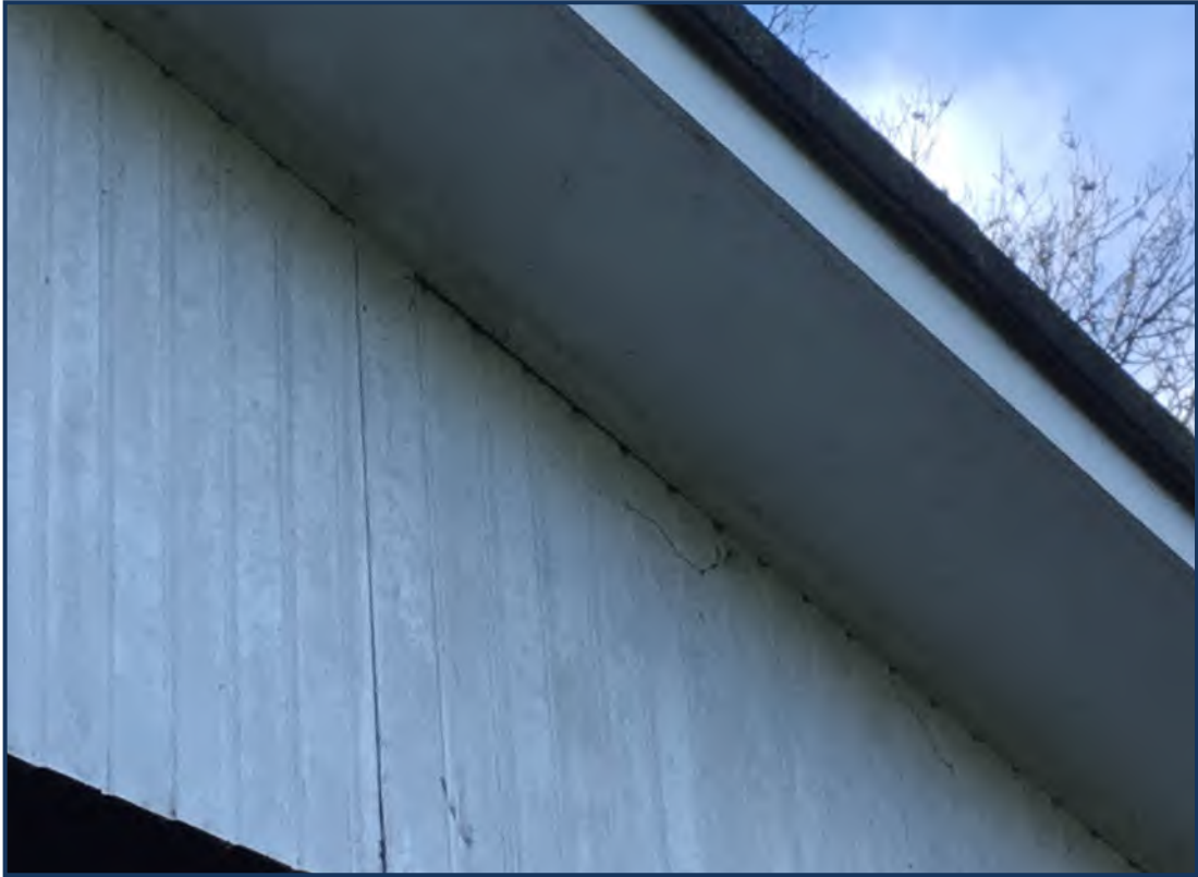
PHOTOGRAPH 11: Building B2 - Gaps in Gable Facade
