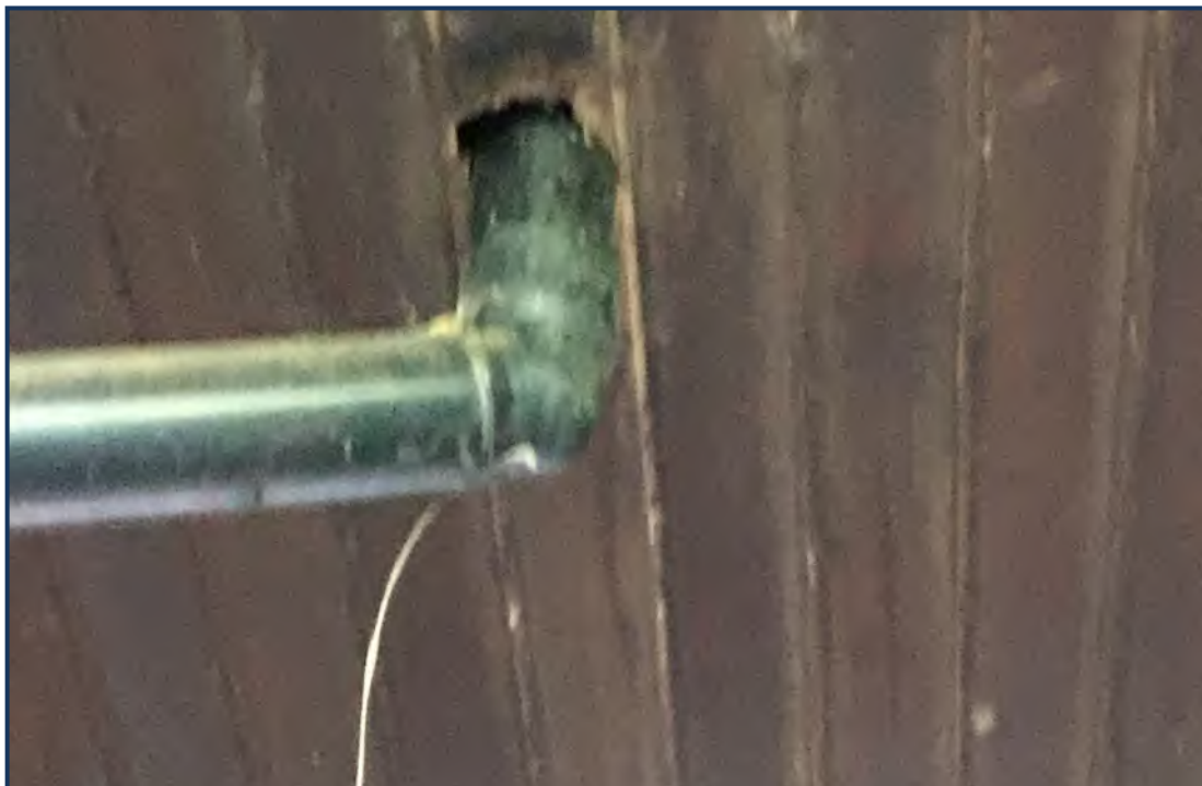
PHOTOGRAPH 10: Building B1 - Gap near Pipe
