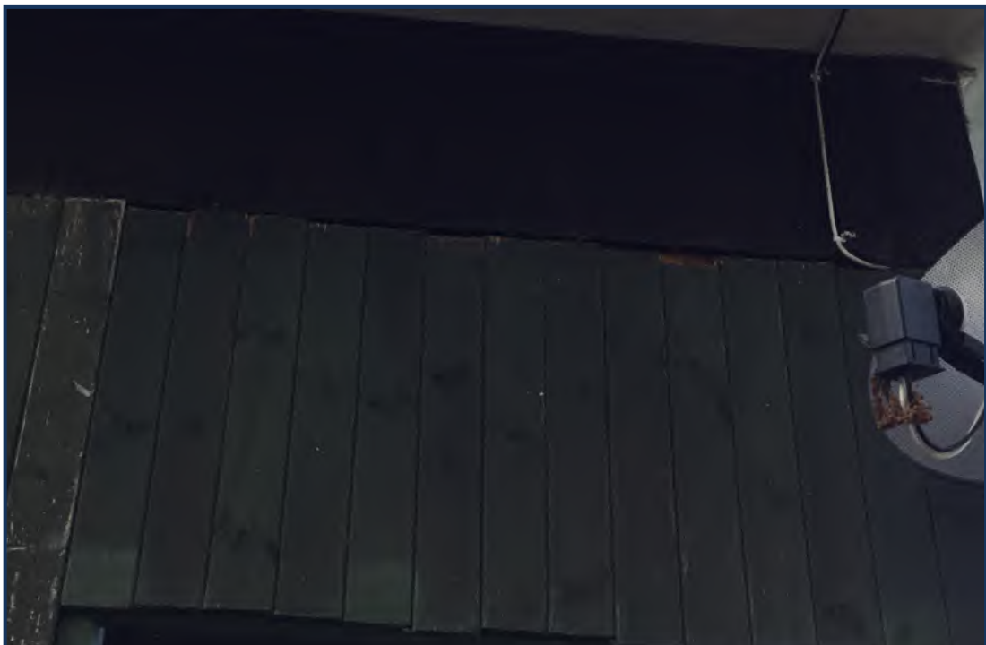
PHOTOGRAPH 12: Building B2 - Gap between External Wall and Barge Board
