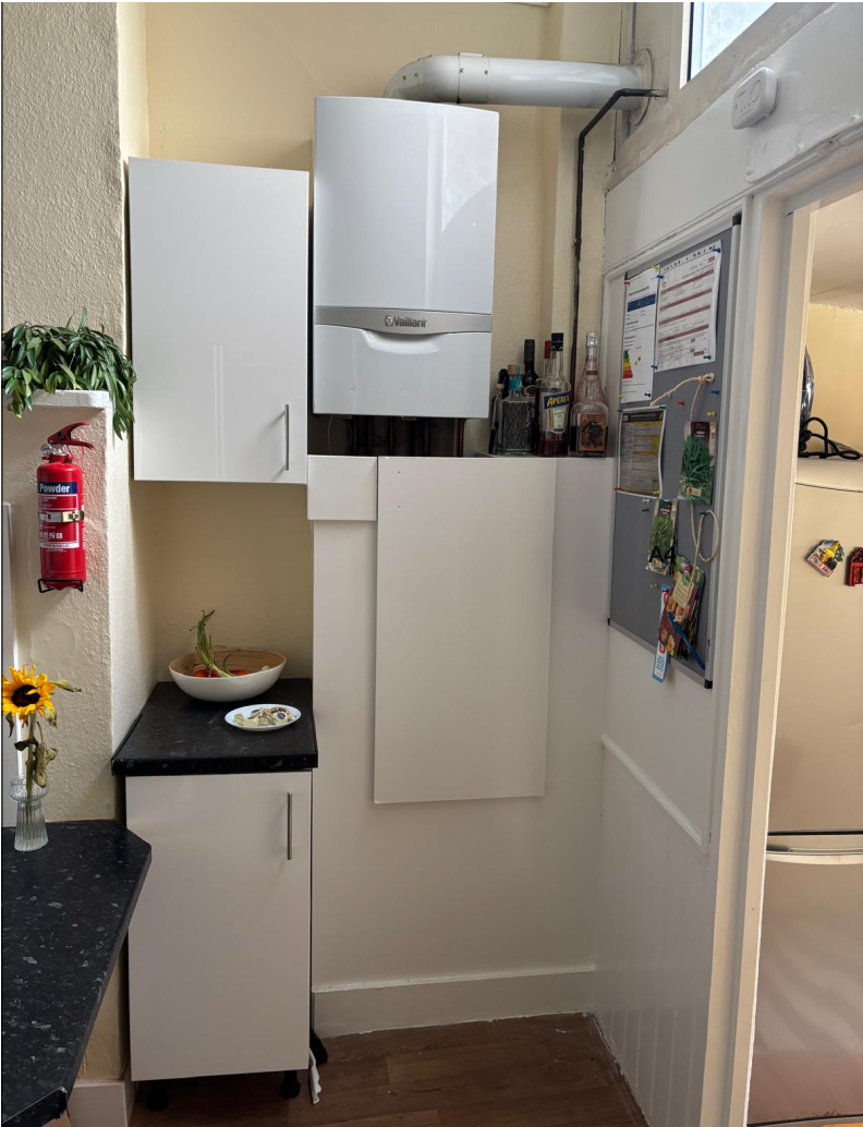
PH2 - New cabinet next to boiler in the kitchen
