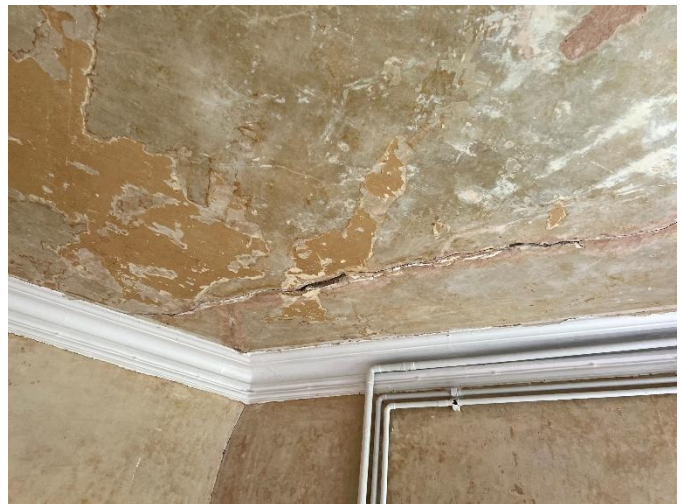
22 Deteriorated lath and plaster ceiling finish with cracking and localised failure. Repairs should retain surviving historic plaster wherever practicable.
