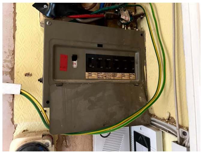
60 Existing older-style consumer unit and associated electrical installation located adjacent to the flat entrance. The installation appears dated in character and likely predates current wiring regulations. Replacement of the consumer unit, associated protective devices and incoming electrical tails is considered reasonable as part of the proposed refurbishment works, subject to confirmation of supply capacity and compliance by a qualified electrical contractor.
