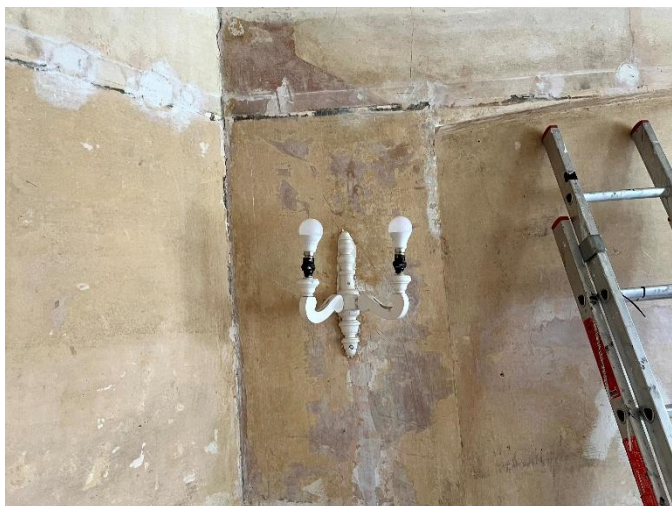
47 Areas of historic wall disturbance and previous electrical installations. Existing service routes should be reused where practicable during refurbishment works.
