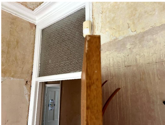
57 Note. Kitchen doors are not fire compliant and likely require upgrading to comply with current regs.
