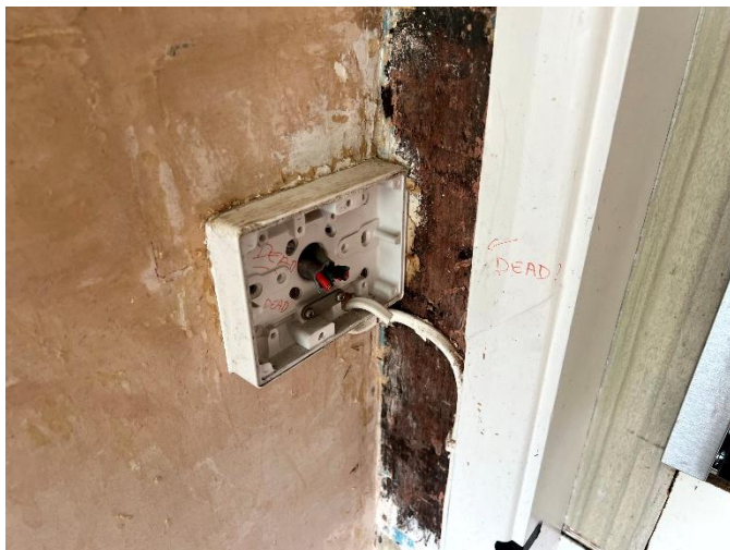
17 Redundant electrical outlet and exposed service chasing to historic wall construction. Illustrates cumulative impact of piecemeal historic alterations to services.
