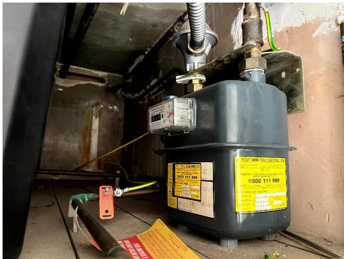
15 Existing gas meter and associated pipework installation. Arrangement appears dated and visually intrusive with limited heritage significance. Proposed rationalisation considered appropriate.
