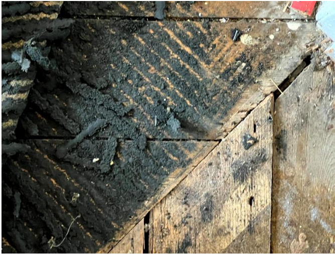
41 Fragmented floorboard junctions and historic service penetrations within original timber floor structure. Comparable to defects identified within approved Flat 18 refurbishment works.
