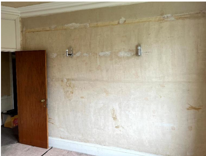
33 Wall elevations showing evidence of historic service routes and previous fittings. Existing plaster finishes appear heavily disturbed by historic interventions.
