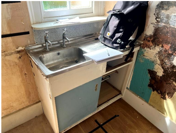
19 Existing kitchen sink arrangement with evidence of localised moisture deterioration and defective finishes to adjacent wall surfaces. Supports proposed kitchen replacement works.
