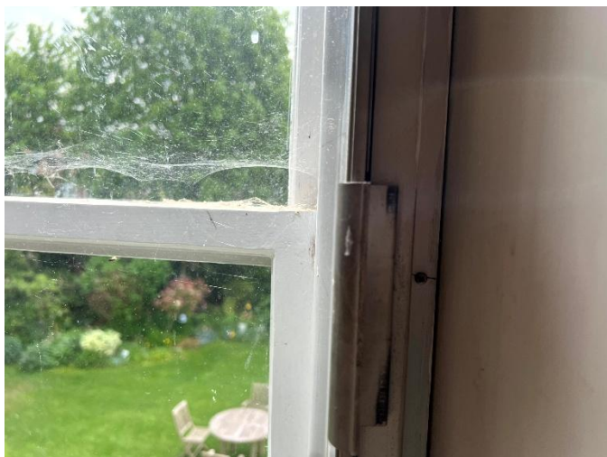
37 Original timber window frame and secondary glazing detail. Window exhibits age-related deterioration but remains important historic fabric. Secondary glazing should be removed with a more modern sympathetic approach taken.
