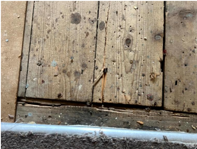
43 Additional view of deteriorated original floorboards with evidence of repeated lifting and disturbance from previous alterations.
