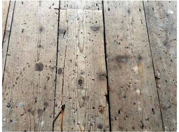
42 General condition of original timber floorboards to bathroom showing age-related abrasion, historic repairs and localised deterioration. Possible woodboring beetle issues previously.
