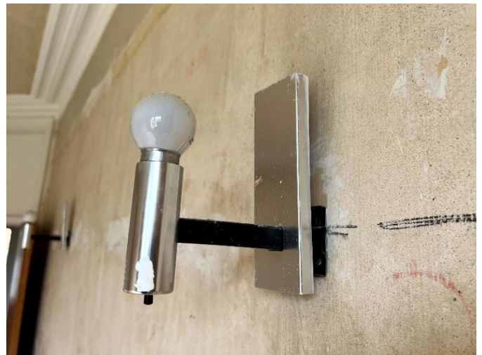
34 Later wall-mounted light fitting fixed to historic plaster wall. Proposed electrical upgrades should minimise further disturbance to original fabric.
