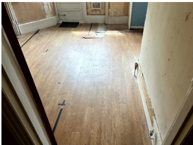
11 Non original laminate flooring with evidence of repeated disturbance associated with previous service installations and alterations throughout.
