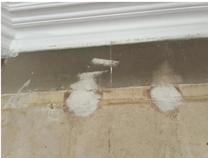
35 Localised plaster repairs and historic fixings beneath cornice line. Evidence of previous alterations and removal of earlier features.
