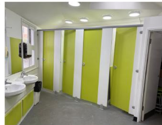
Fig. 9 Washroom fittings proposed for replacement in room CH114
